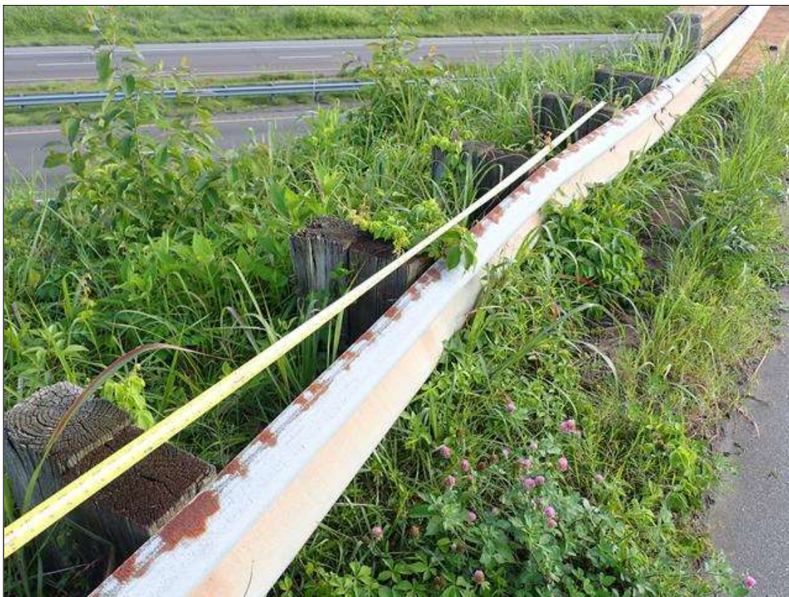
(PAR) southwest guardrail, 15 feet from bridge, impact damage (10 feet)
