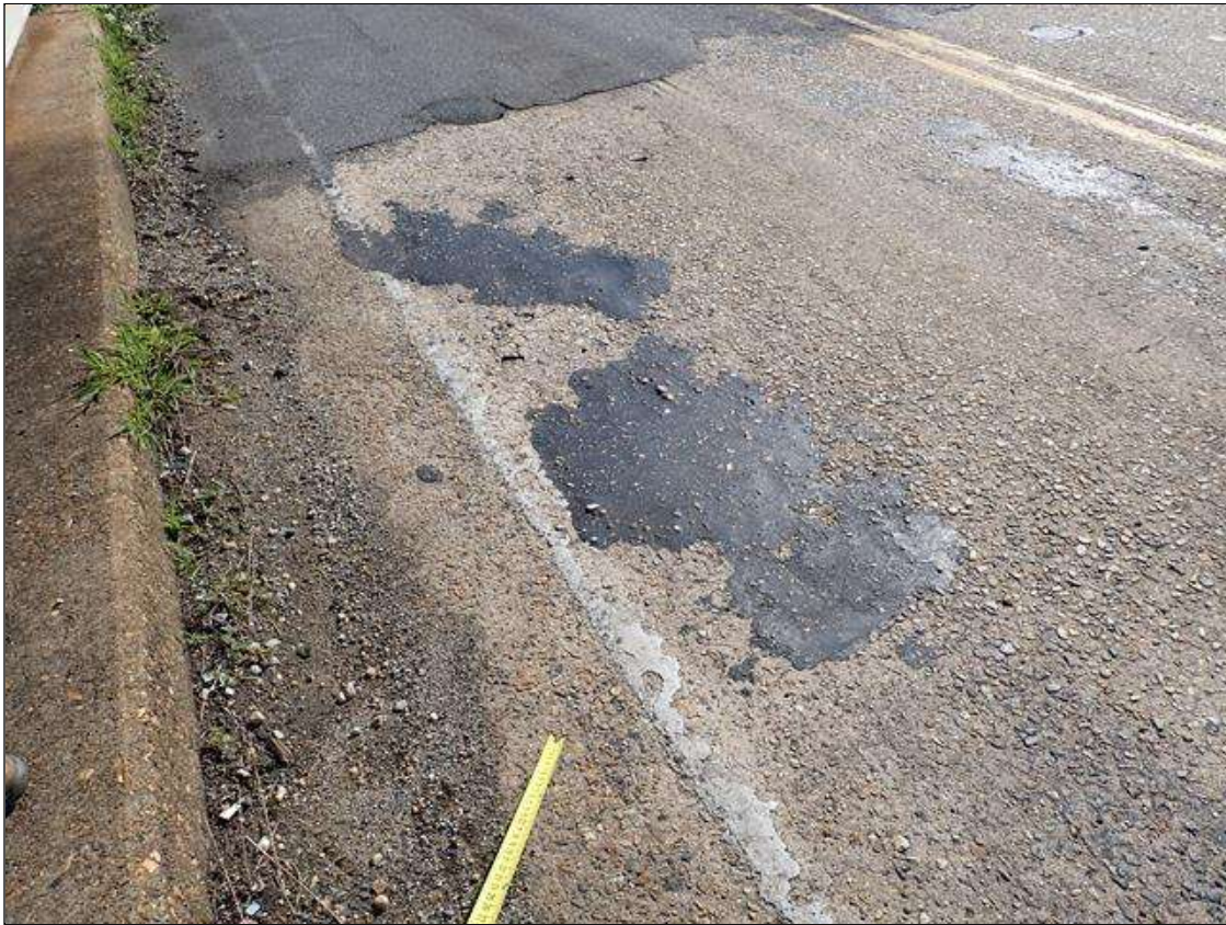
Span 4 Deck: SPAN 4 TOP OF DECK HAS SCATTERED sound and unsound PATCHES [up to 2 foot diameter x up to 1/2 inch deep]
