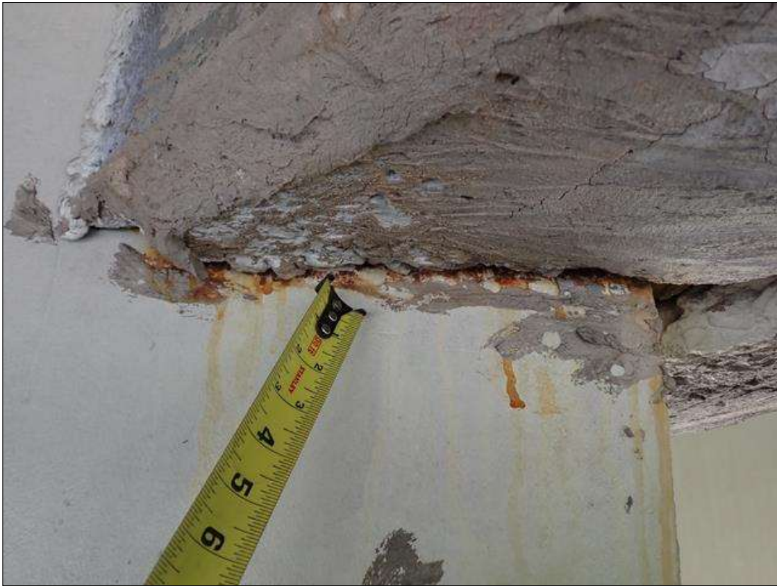
Span 2 Beam 2: (PAR) at bent 2, web adjacent to diaphragm, painted over section loss (5/16 inch average remaining x 9 inch x 1 inch) with corrosion reinitiated
