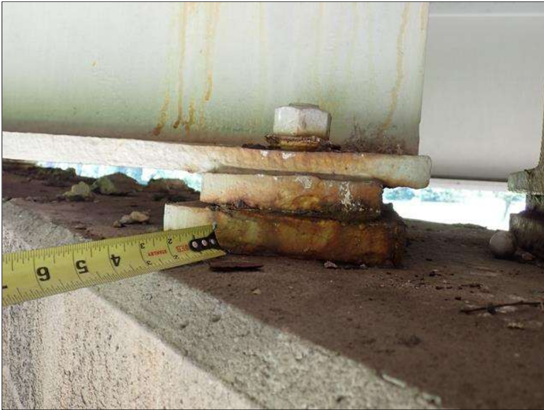
Span 2 Beam 3 - Far Bearing 3: painted over section loss (up to 1/8 inch deep) with corrosion reinitiated; pack rust
