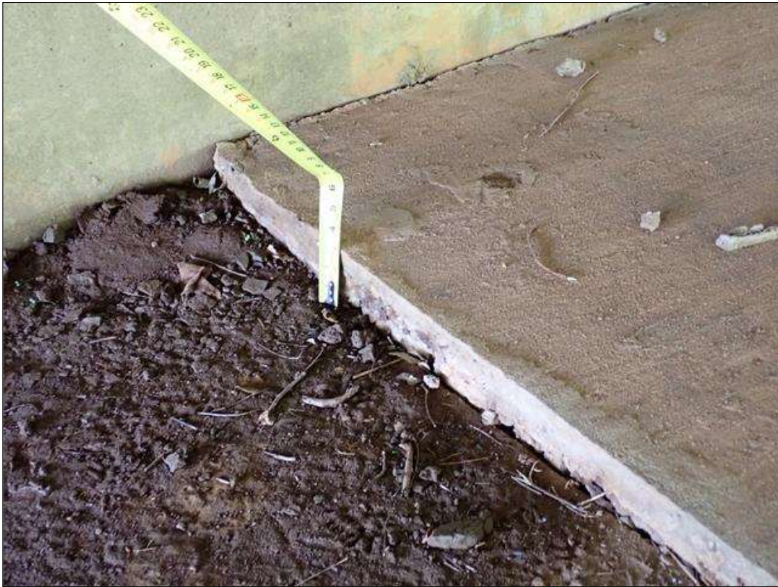
end bent 2 slope protection, in bay 1, near cap, settlement (up to 3 inches) with adjacent longitudinal crack (up to 1/8 inch x 10 feet)
