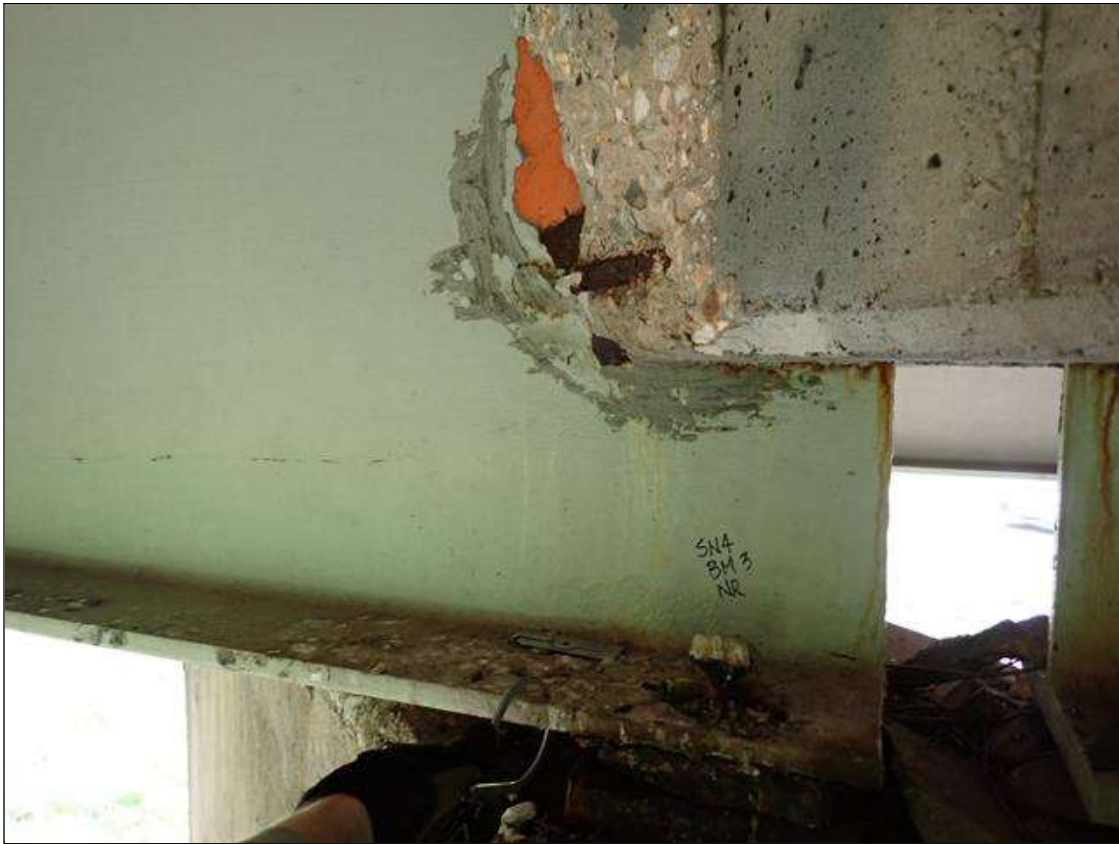
Span 4 Beam 3: (PAR) at bent 3, web adjacent to diaphragm, corrosion with section loss (5/16 inch average remaining x 14 inch x 6 inch); painted over section loss: lower web (3/8 inch average remaining x 1 foot x 2 inches), bottom flange (0.65 inch average remaining x 1 foot)
