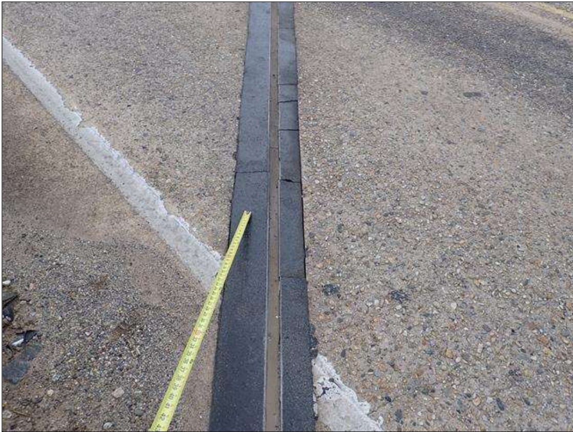
Span 2 Bent 1 Joint: (PAR) spans 1 and 2 header, in both travel lanes, delaminations (up to 12.5 feet x 6 inches) with cracks (up to 1/8 inch) and separated from adjacent deck (up to 1/2 inch)
