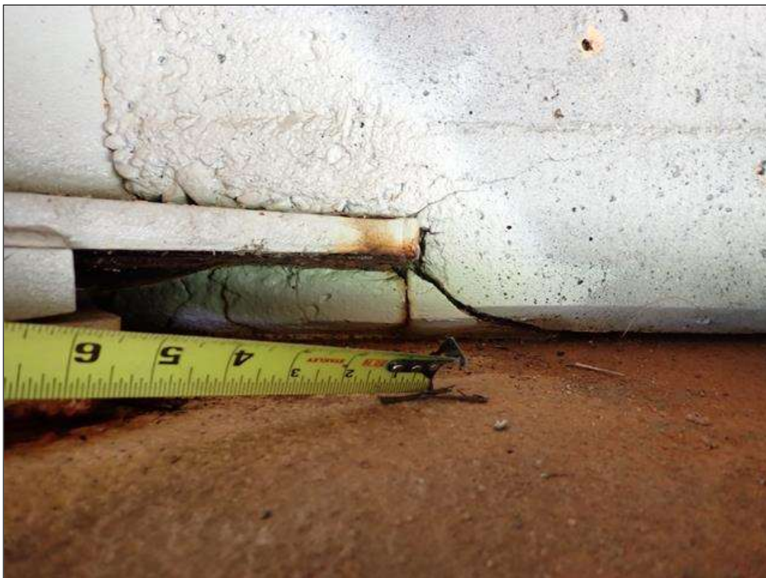
End Bent 1 Abutment: at beam penetrations, spall, up to 9 inch x 4 inch
