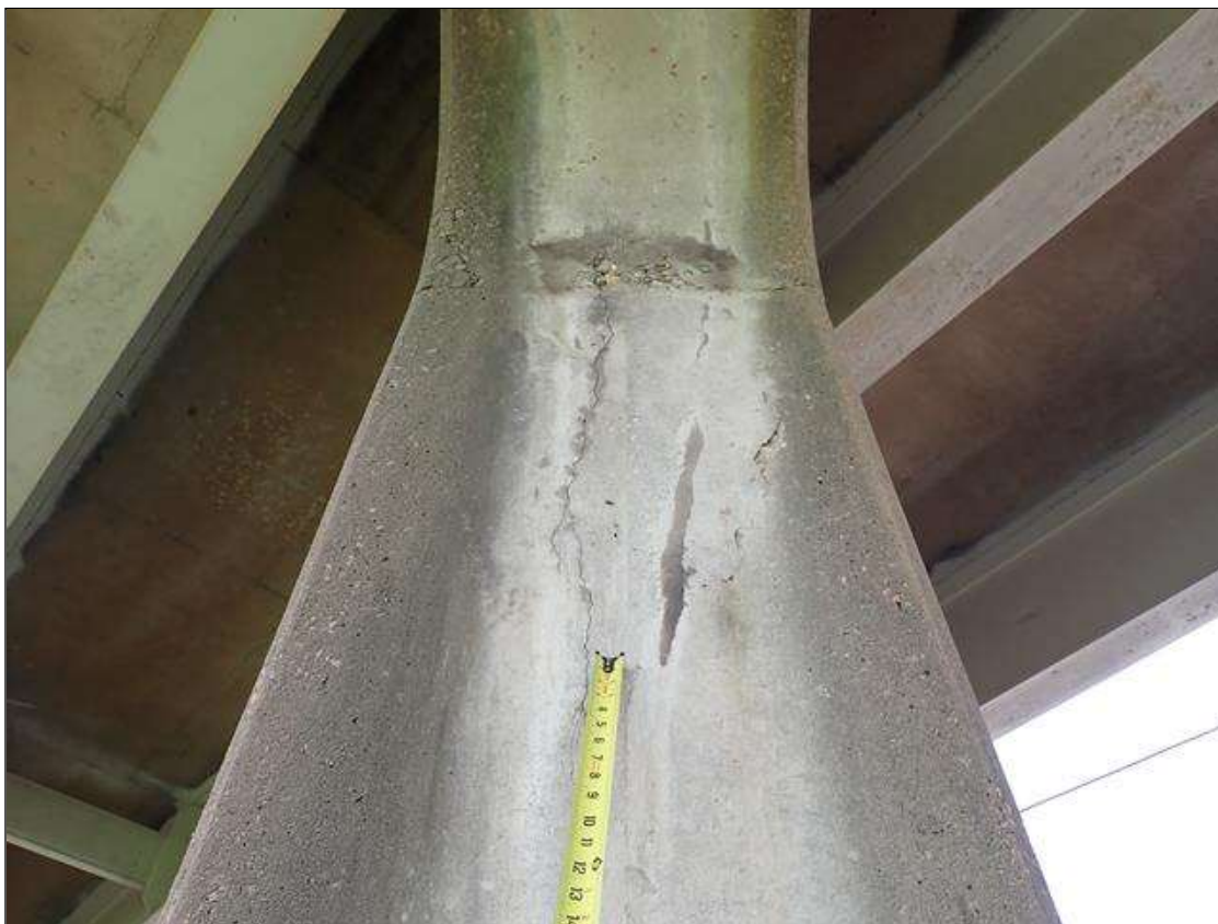
Bent 1 Pile 2: East face under cap, delamination [5 feet x 19 inches]
