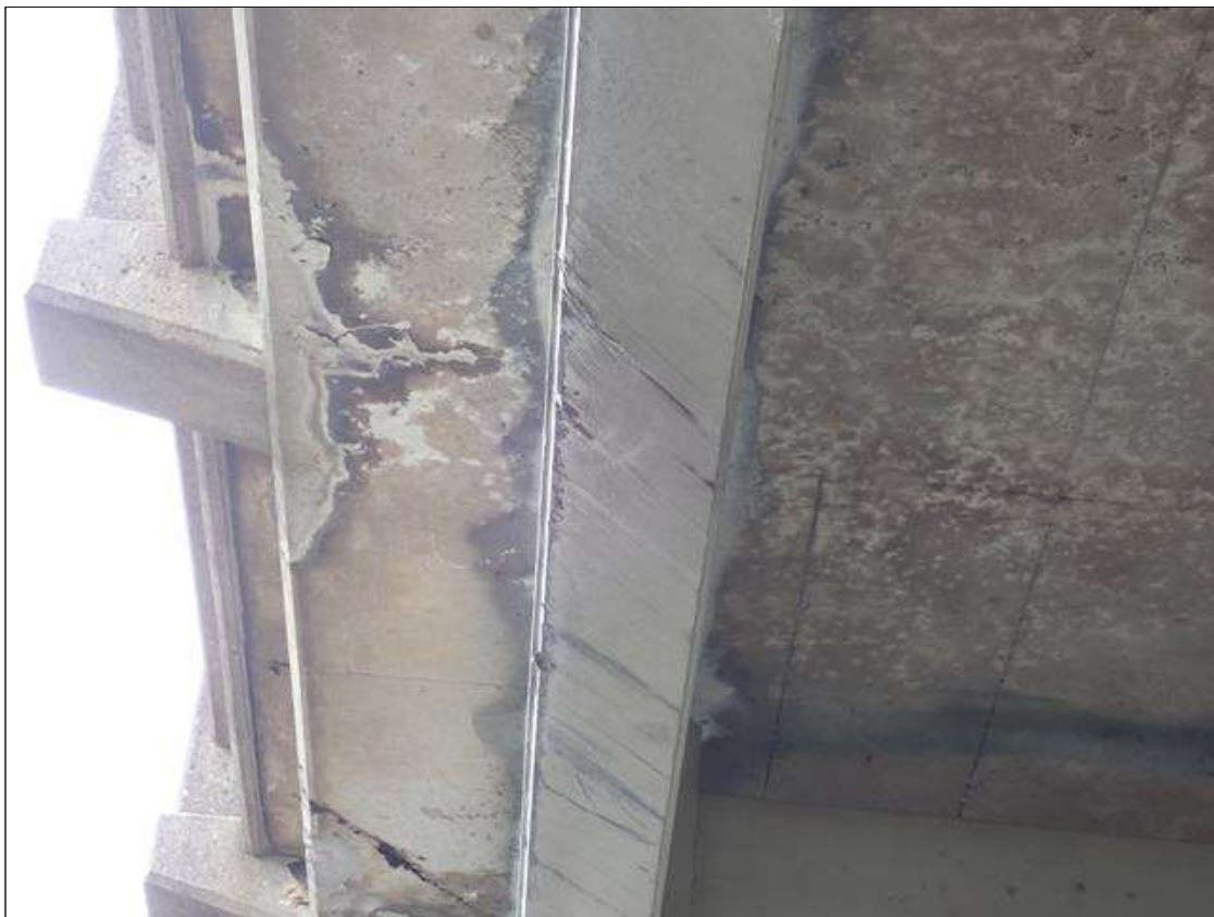
Span 3 Beam 4: (PAR) COVER PLATE OVER RIGHT TRAVEL LANE AND SHOULDER, IMPACT SCRAPES WITH GOUGES (APPROXIMATELY 1/2 INCH DEEP)
