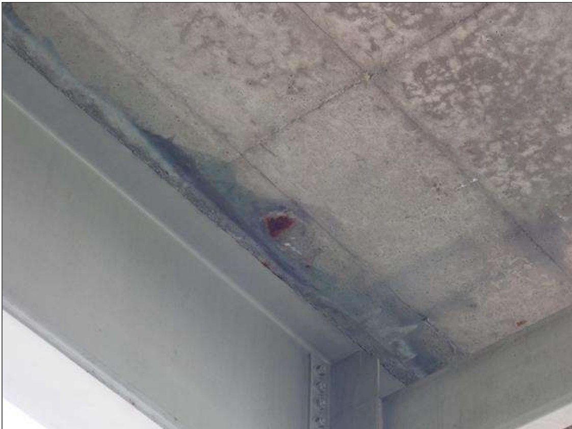
Span 2 Deck: (PAR) bays 2 and 3, adjacent to beams, areas of rust stains at random
