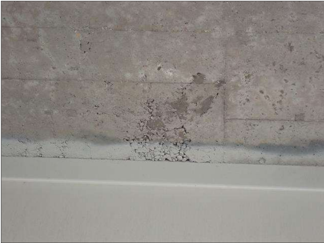
Span 3 Deck: underside of bays 2 and 3, near half of span, areas of poor consolidation (up to 3.5 feet x 15 inch x 1 inch deep)
