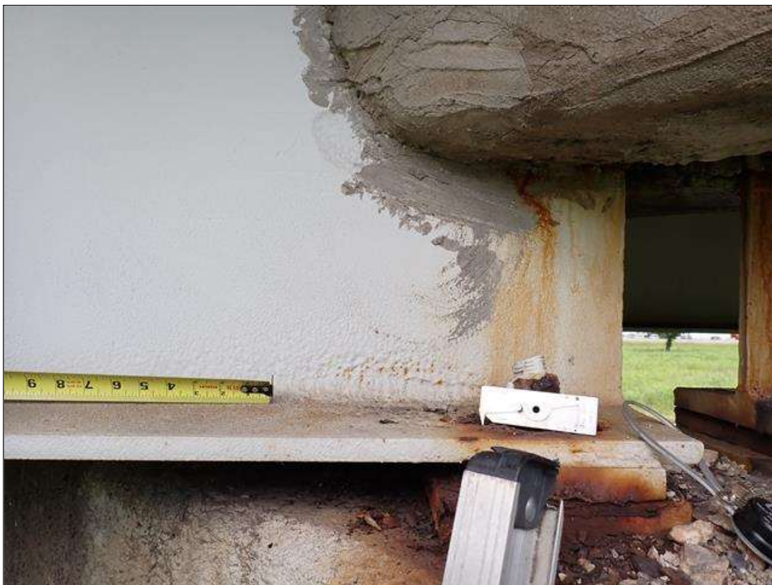
Span 1 Beam 4: (PAR) at bent 1, painted over section loss: web adjacent to diaphragm (5/16 inch average remaining x 12 inch x 3 inch) lower web (5/16 inch average remaining x 10 inch x 2 inch); bottom flange (0.63 inch average remaining x 6 inches) with corrosion reinitiated
