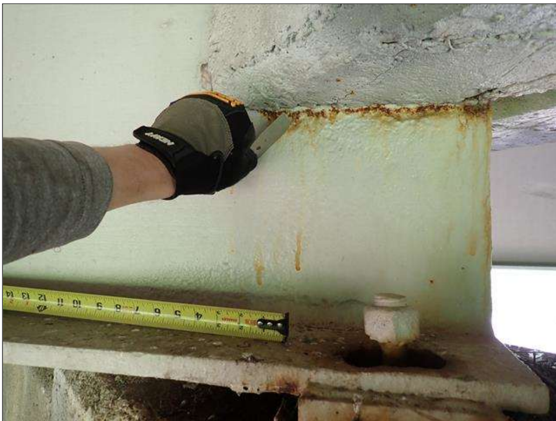
Span 1 Beam 2: (PAR) at bent 1, painted over section loss: web at end diaphragm (5/16 inch average remaining 12 inches long x up to 2 inches wide) with reactivated surface corrosion; lower web (3/8 inch average remaining x 15 inch x 3 inch)
