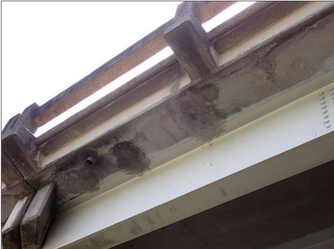
Span 1 Deck: SPAN 1 BOTTOM OF DECK IN WEST OVER HANG HAS SCATTERED PATCHED AREAS. APPROXIMATELY 20 SQUARE FEET.
