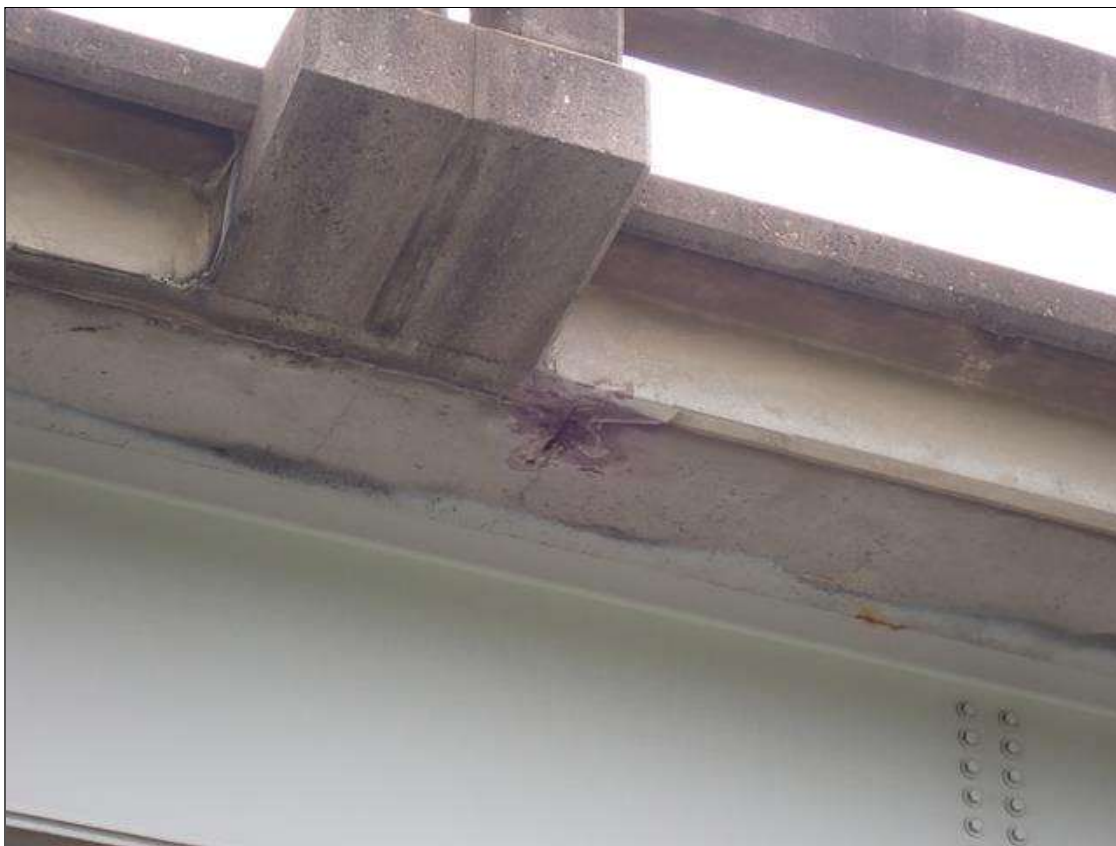
Span 3 Deck: (PAR) left overhang near mid span, spall [8 inch x 4 inch x 1 inch deep] with exposed rusted reinforcing [no measurable loss]
