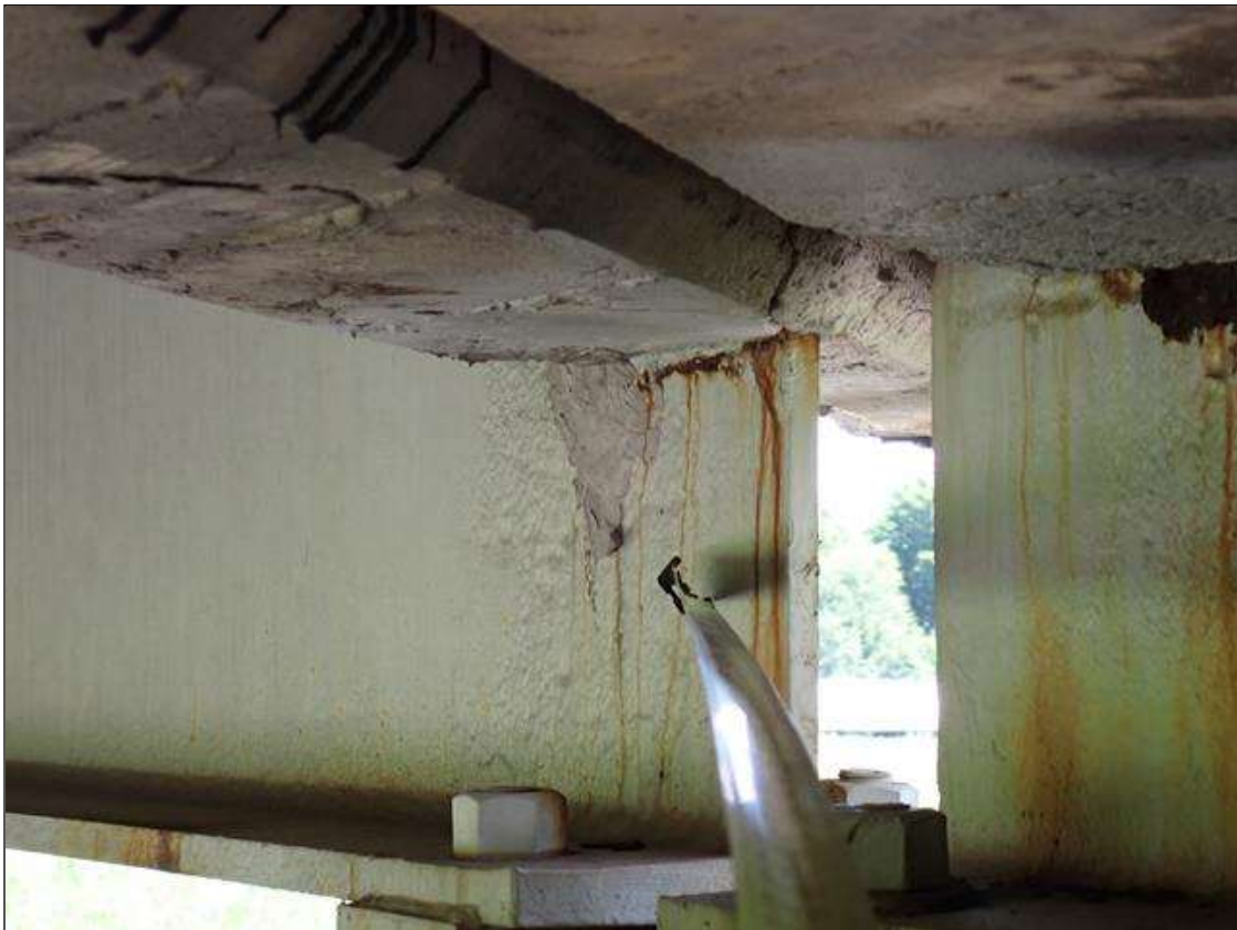
Span 3 Beam 4: (PAR) at bent 2, web adjacent to diaphragm, painted over section loss (5/16 inch average remaining x 12 inch x 6 inch); lower web, painted over pitting (up to 1/8 inch deep x 1 foot x 3 inches) with corrosion reinitiated
