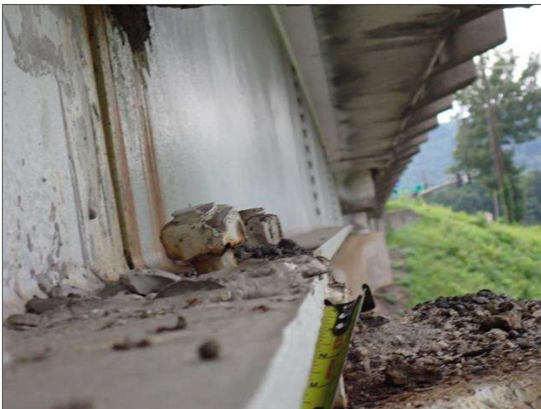
Span 4 Beam 1 - Near Bearing 1: rust scale; both anchor bolts (approximately 10 percent section loss)
