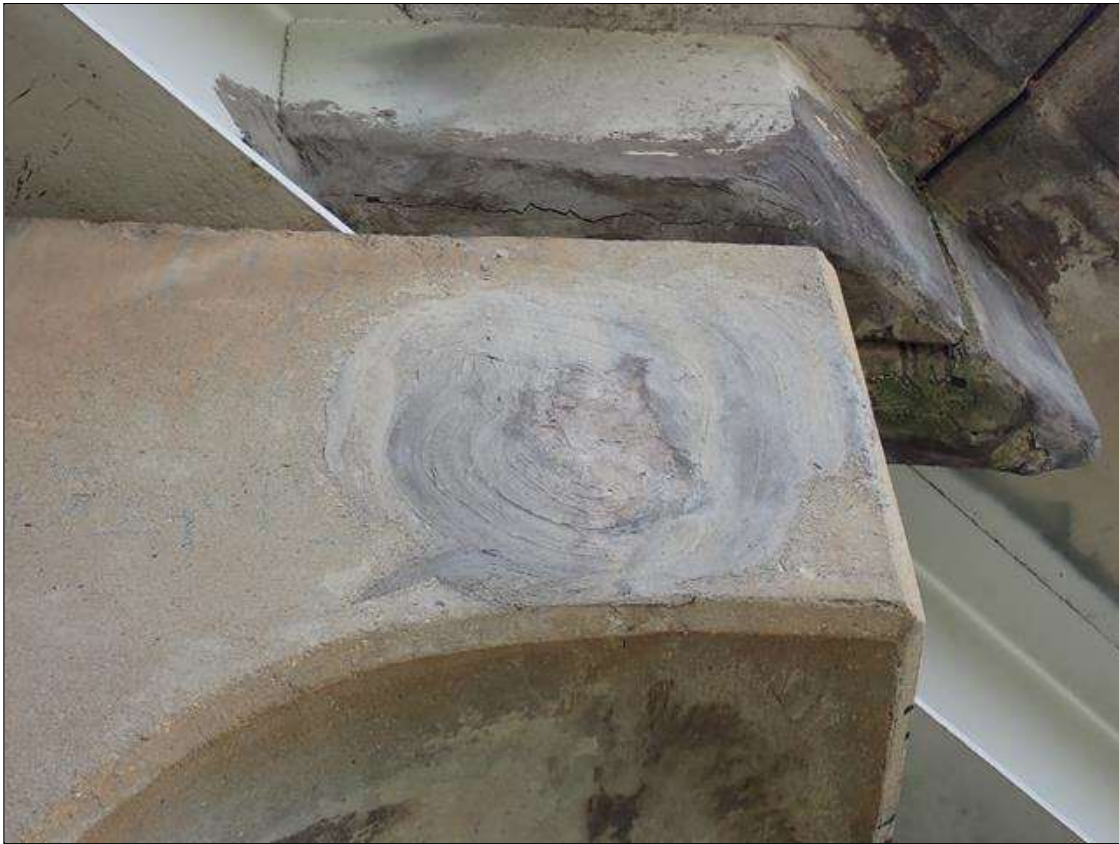
Bent 2 Cap 1: BENT 2 NORTH FACE OF CAP HAS AN UNSOUND PATCHED AREA (2 FEET X 15 INCH) WEST SIDE OF BEAM 1.
