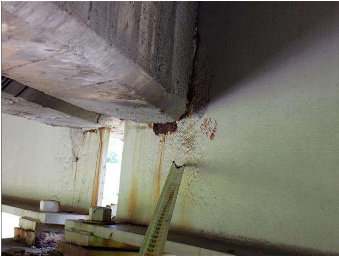
Span 2 Beam 4: (PAR) at bent 2, web adjacent to diaphragm, painted over section loss (1/4 inch average remaining x 14 inch x 8 inch) with adjacent pitting (up to 1/8 inch deep) with corrosion reinitiated
