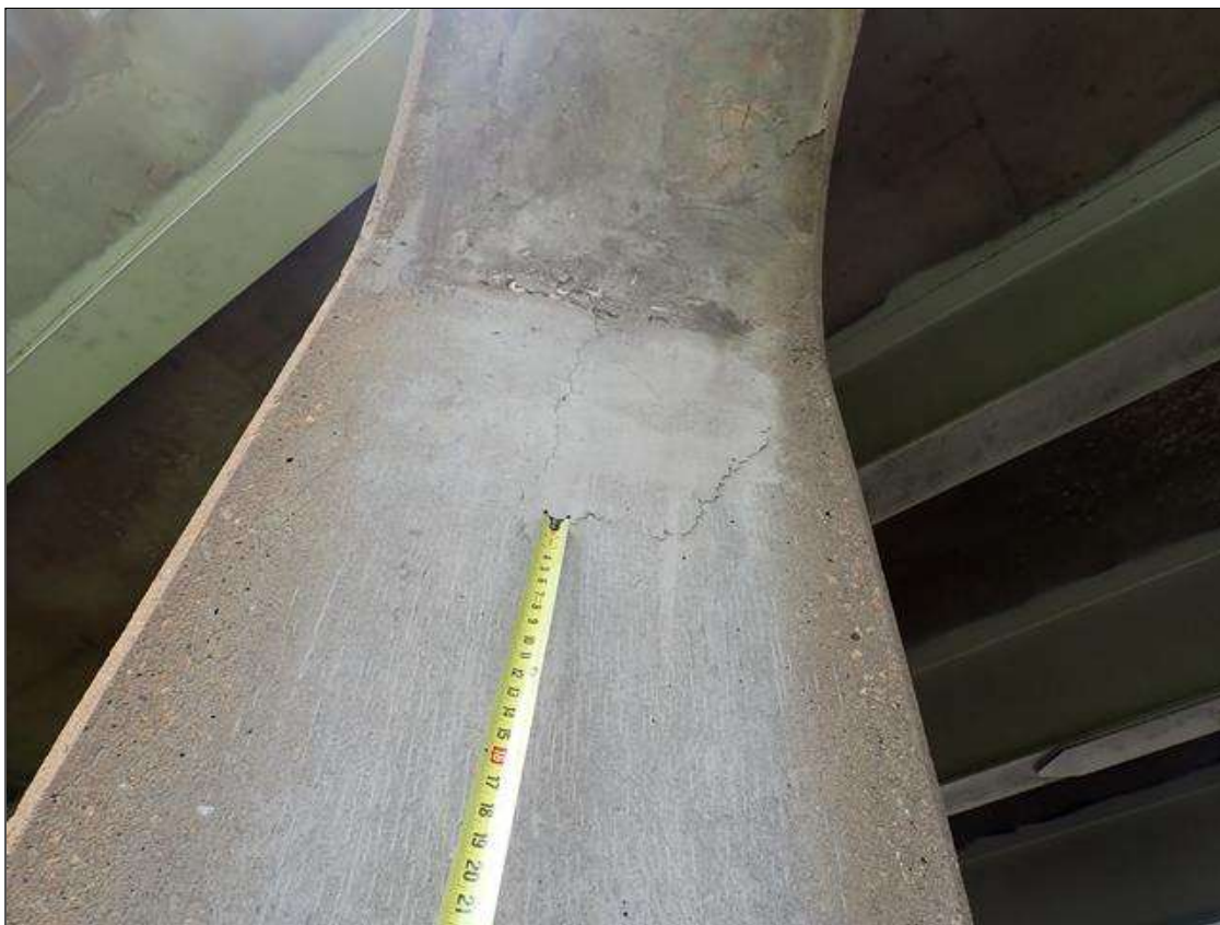
Bent 1 Pile 3: on East and West faces of pile, delaminations [up to 18 inch x 1 foot]
