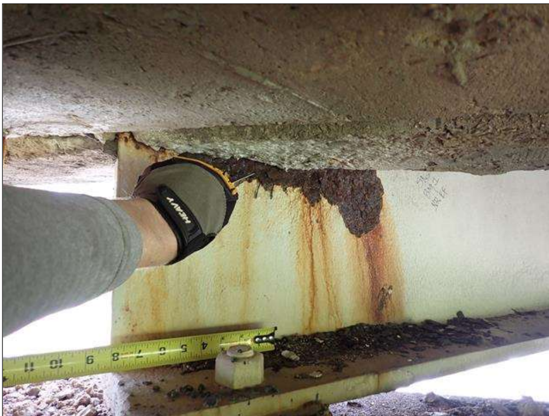
Span 2 Beam 1: (PAR) at bent 1, web adjacent to diaphragm, corrosion with section loss (1/4 inch average remaining x 15 inch x 7 inch); painted over pitting: lower web (up to 1/16 inch deep x 3 feet x 6 inches), bottom flange (1/8 inch deep x 2 feet)
