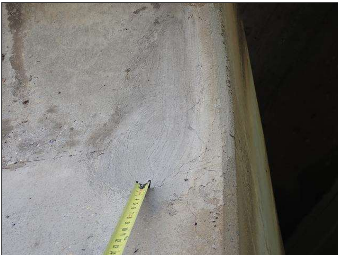
Bent 2 Pile 1: West face below cap, sound patch [8 inch x 2 feet] with cracks [up to 1/32 inch]
