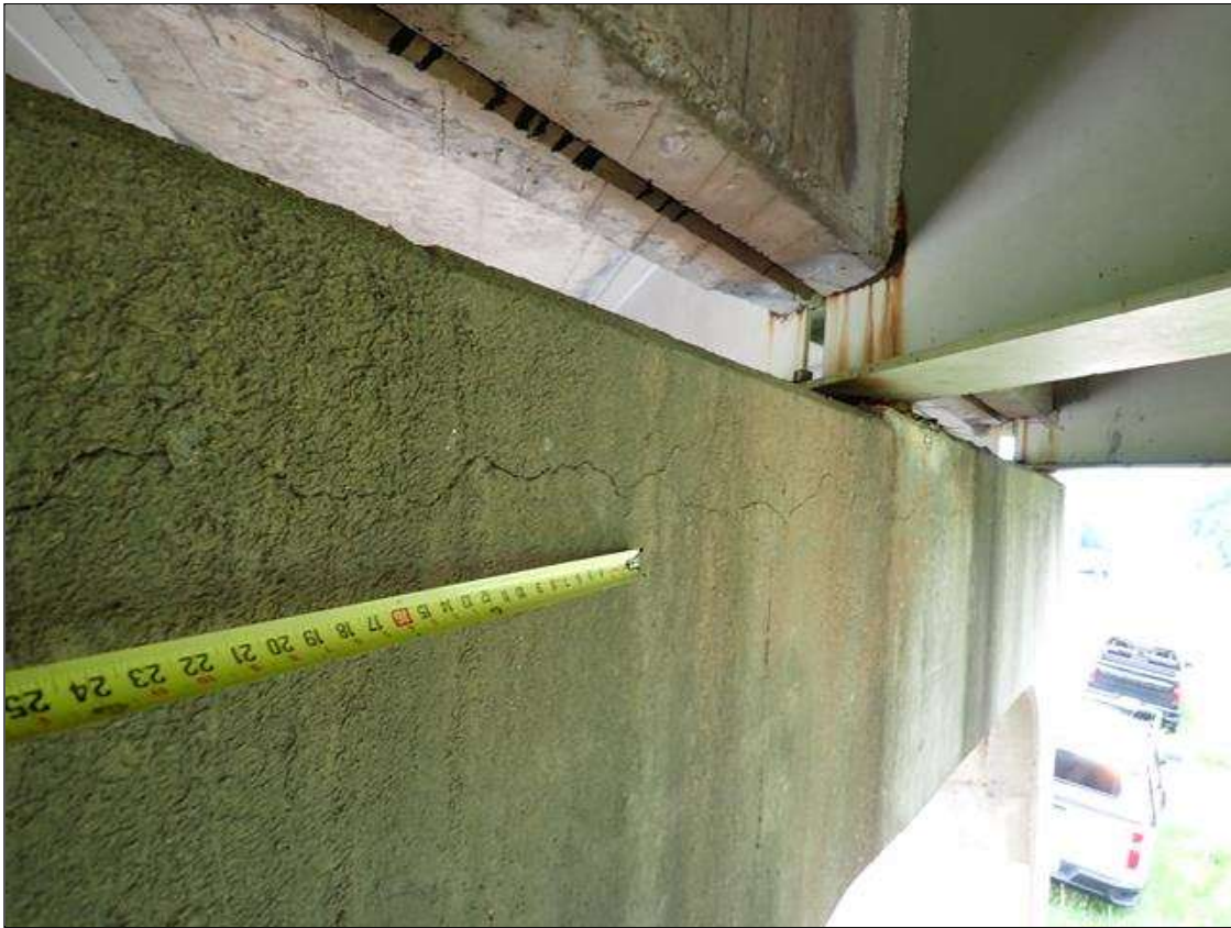
Bent 3 Cap 1: north face, below bays 1 and 2, longitudinal crack (up to 1/16 inch x 20 feet)
