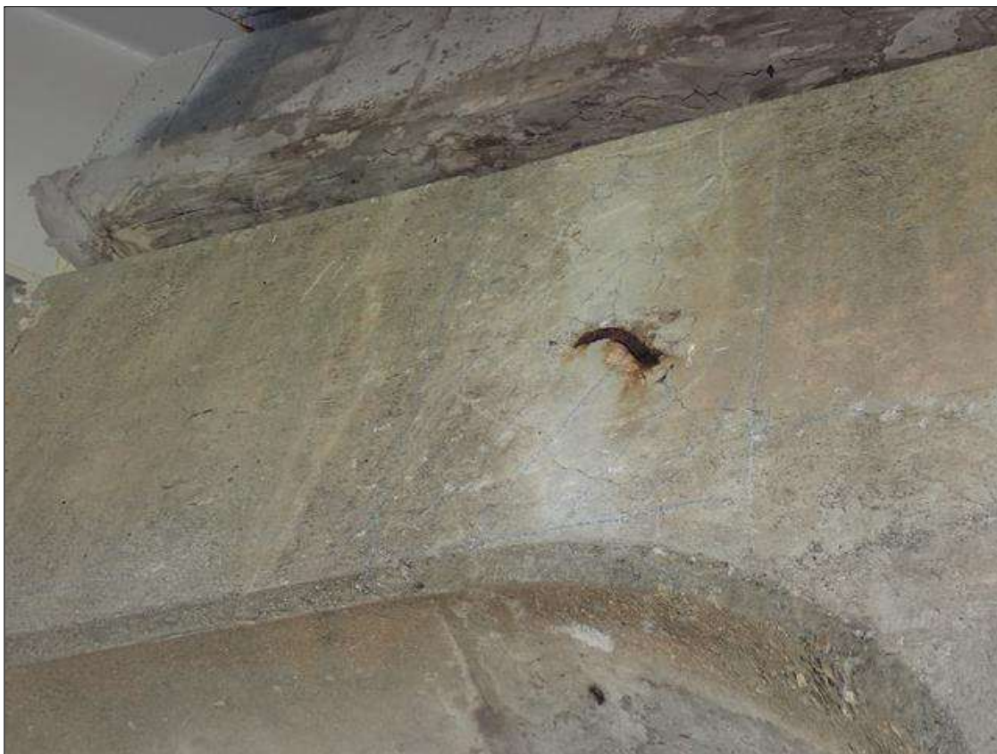
Bent 2 Cap 1: south and north faces of cap, multiple delaminations/spalls (up to 8 feet x 2 feet x 1.5 inch deep), some with exposed rusted rebar and associated cracks (up to 1/8 inch wide)
