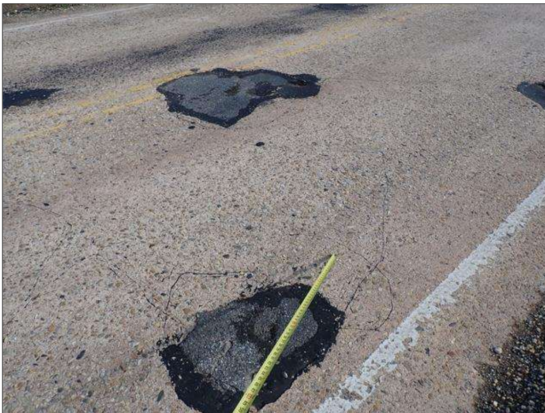
Span 3 Deck: (PAR) SPAN 3 TOP OF DECK HAS SCATTERED sound and unsound PATCHES [up to 8 feet x up to 4 feet x up to 1.5 inches deep] some with depressions; with adjacent spalls/delaminations (up to 1.5 foot diameter x 1.5 inches deep)
