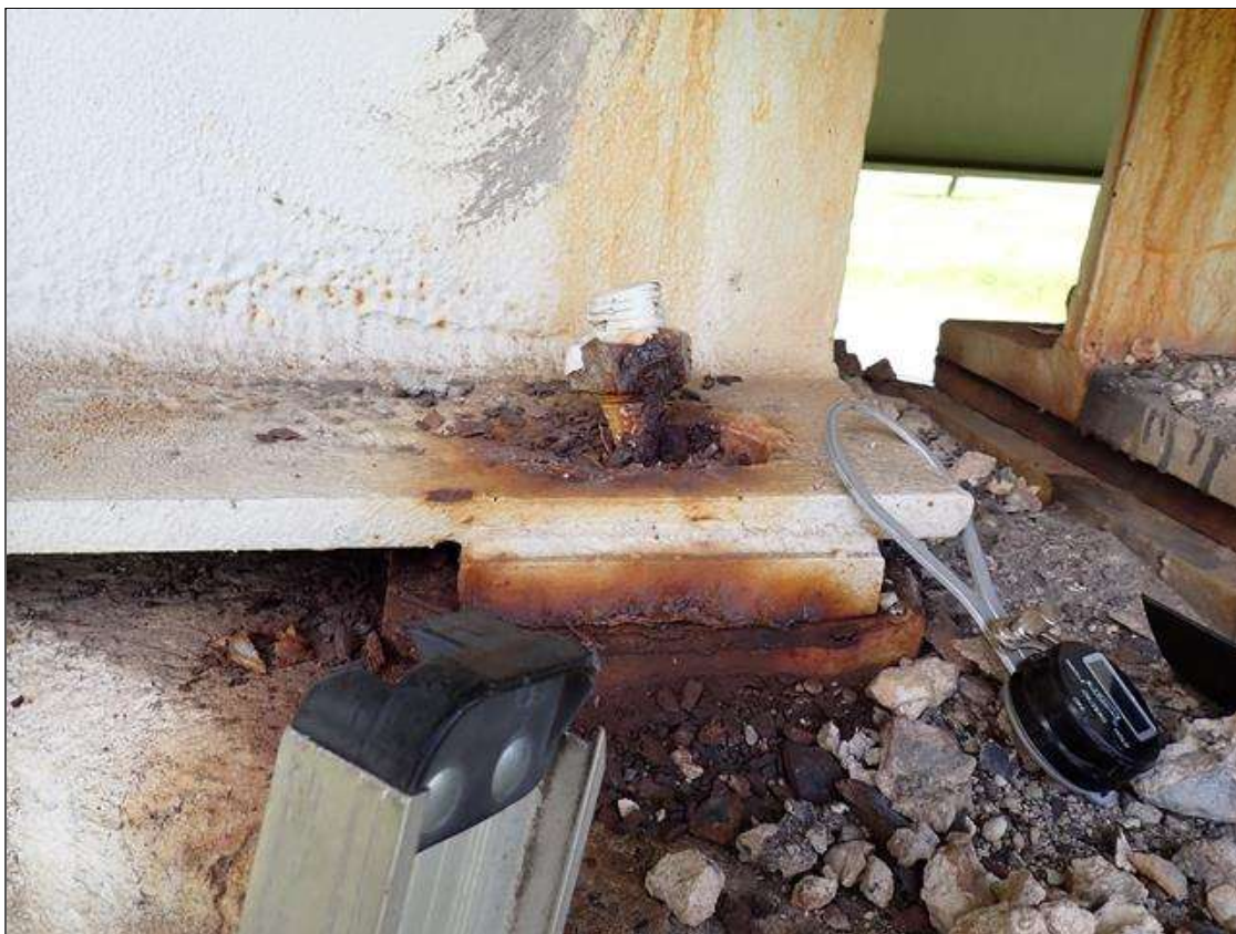
Span 1 Beam 4 - Far Bearing 4: (PAR) corrosion with section loss (up to 1/8 inch); right anchor bolt (50 percent average remaining)
