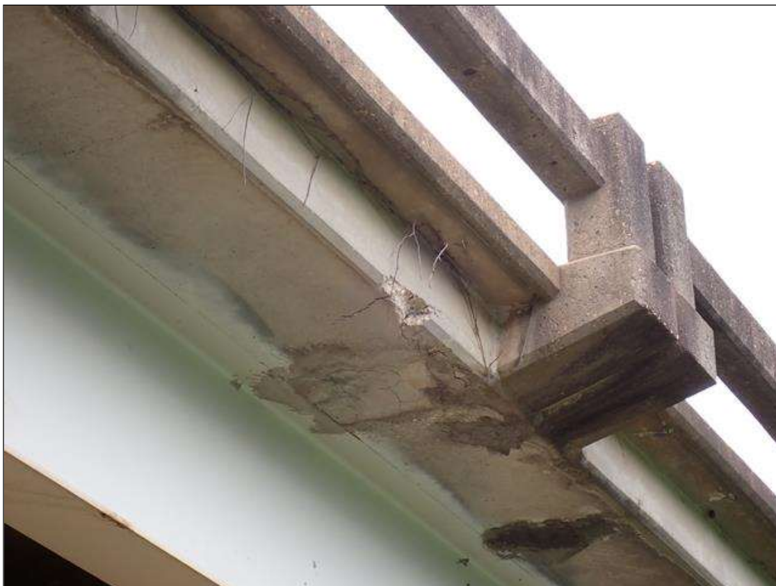
Span 4 Deck: underside right overhang at midspan, spall with adjacent delamination, 34 inch x 18 inch x 2 inch deep
