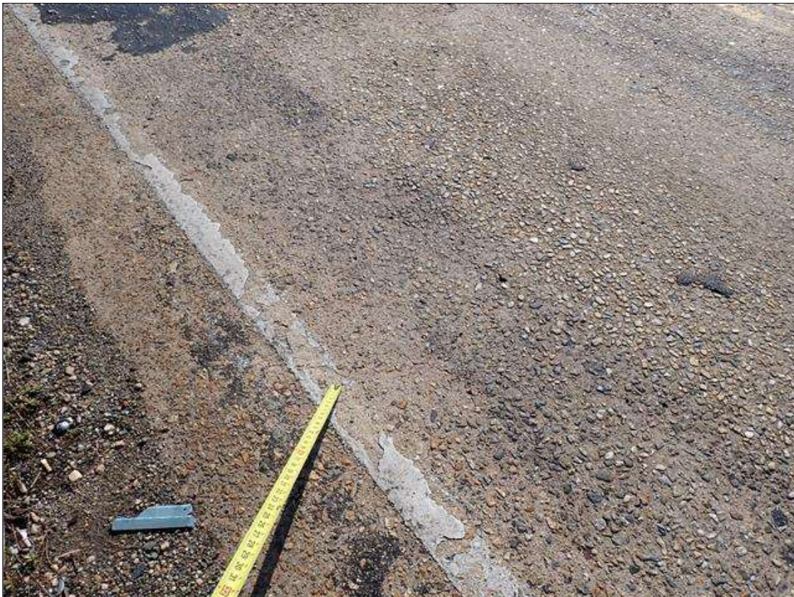
Span 4 Deck: SPAN 4 TOP OF DECK HAS MAP CRACKING UP TO 1/16 INCH AND COARSE AGGREGATE EXPOSED THROUGH OUT.
