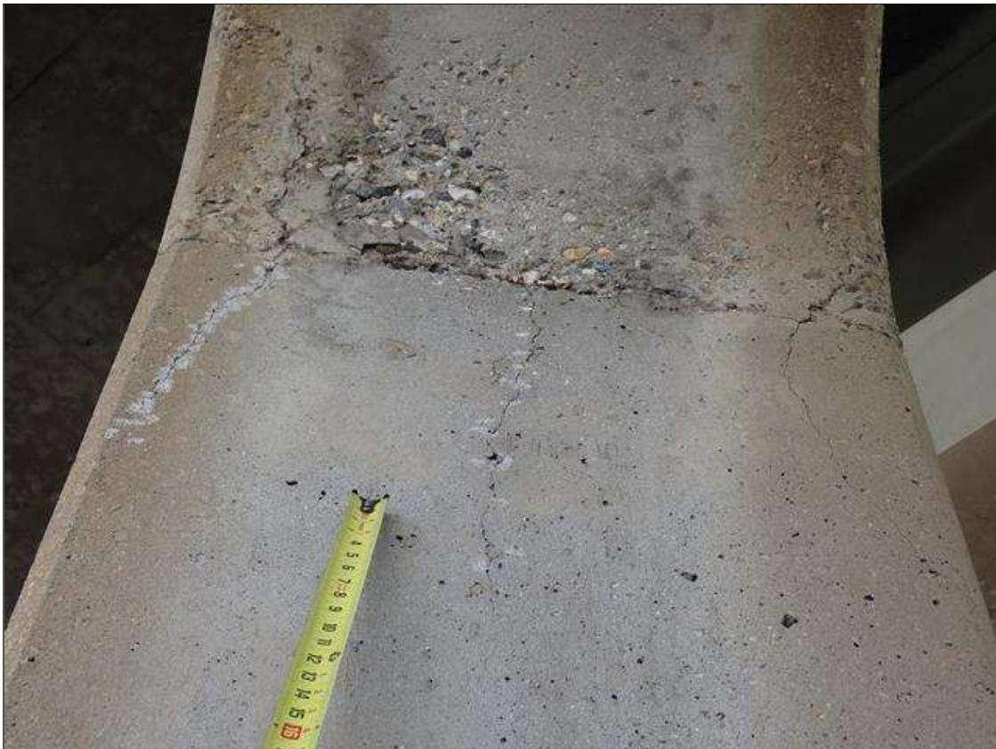
Bent 2 Pile 2: West and East faces, delamination [up to 14 inch x 11 inch] with associated map cracking up to 1/32 inch with efflorescence
