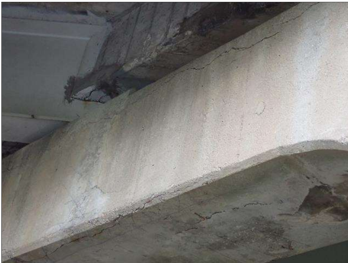
Bent 3 Cap 1: south face, upper and lower edges, longitudinal cracks (up to 1/8 inch x full length) with adjacent delaminations (up to 8 feet x 8 inch)
