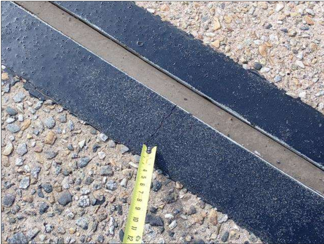
Span 4 Bent 3 Joint: along the headers, transverse cracks (up to 1/32 inch x 6 inches) at random
