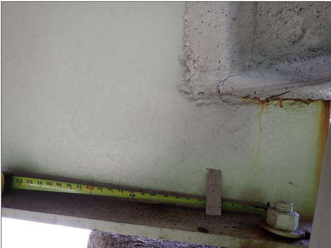
Span 1 Beam 1: (PAR) at bent 1, painted over section loss: web adjacent to diaphragm (5/16 inch average remaining x 12 inch x 5 inch); lower web (7/16 inch average remaining x 15 inches x 2 inches) with corrosion reinitiated
