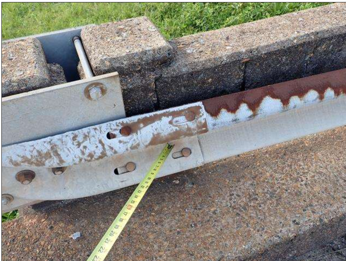
(PAR) southeast guardrail attachment, improper lap
