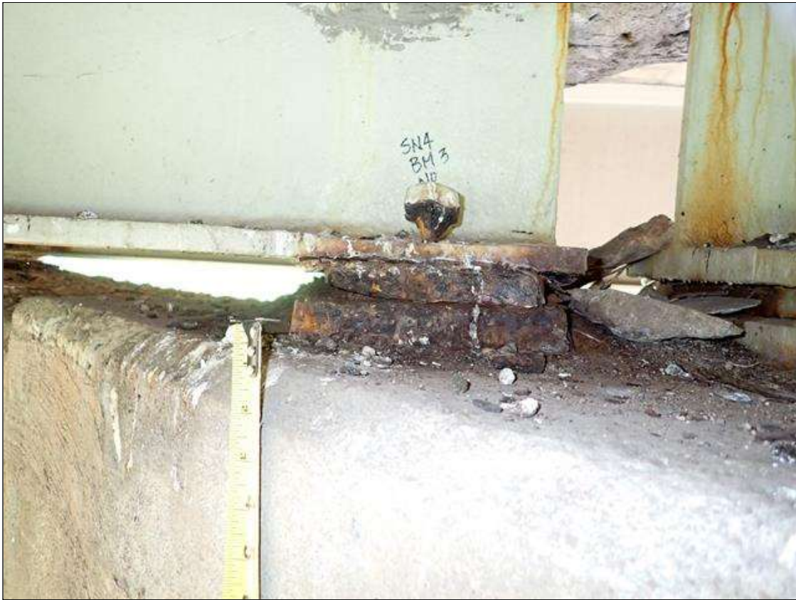
Span 4 Beam 3 - Near Bearing 3: (PAR) corrosion with section loss (up to 1/4 inch deep); left anchor bolt (75 percent section loss)
