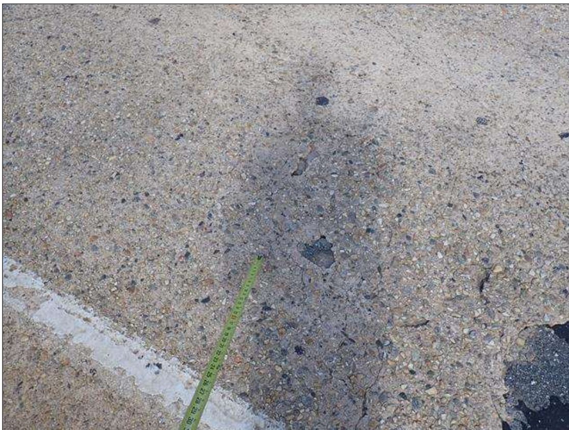
Span 1 Deck: scattered throughout top of deck, multiple spalls/delaminations [up to 18 inches x up to 20 inches x up to 1.5 inches deep] no exposed reinforcing
