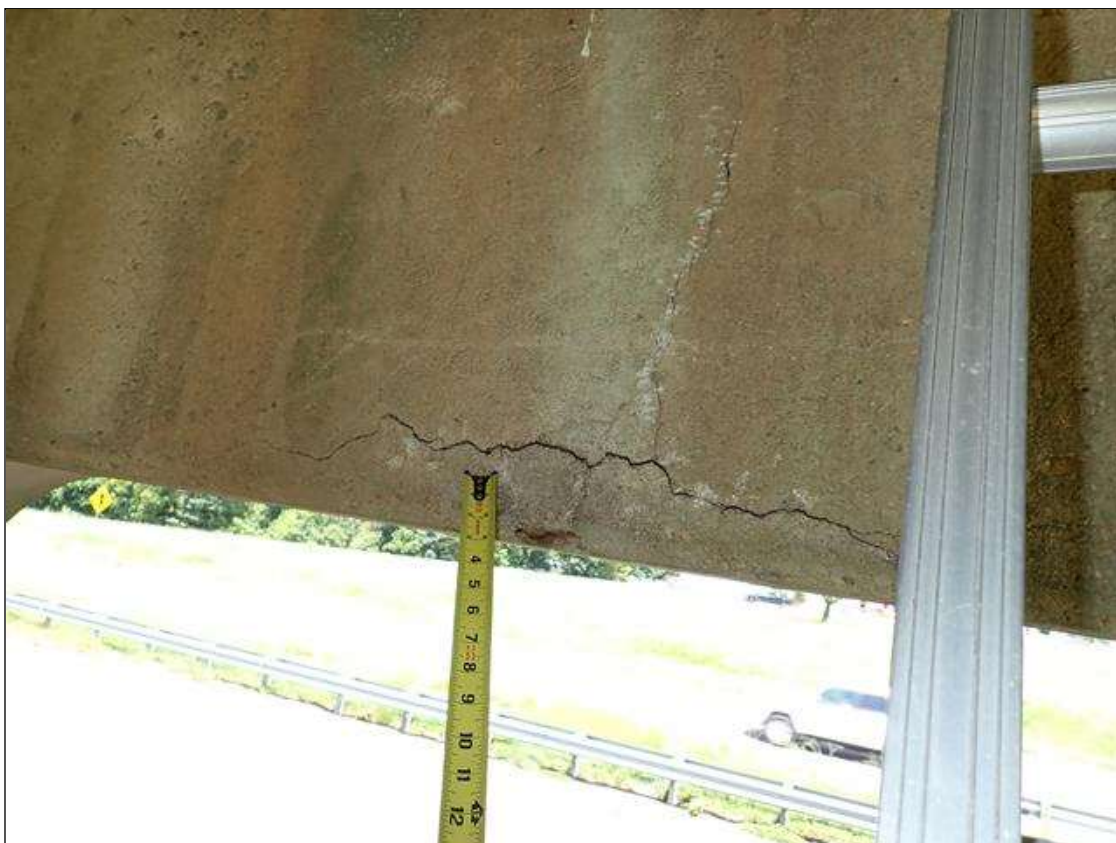
Bent 1 Cap 1: south face, below beams 2 and 3, vertical and longitudinal cracks (up to 1/8 inch x 5 feet)
