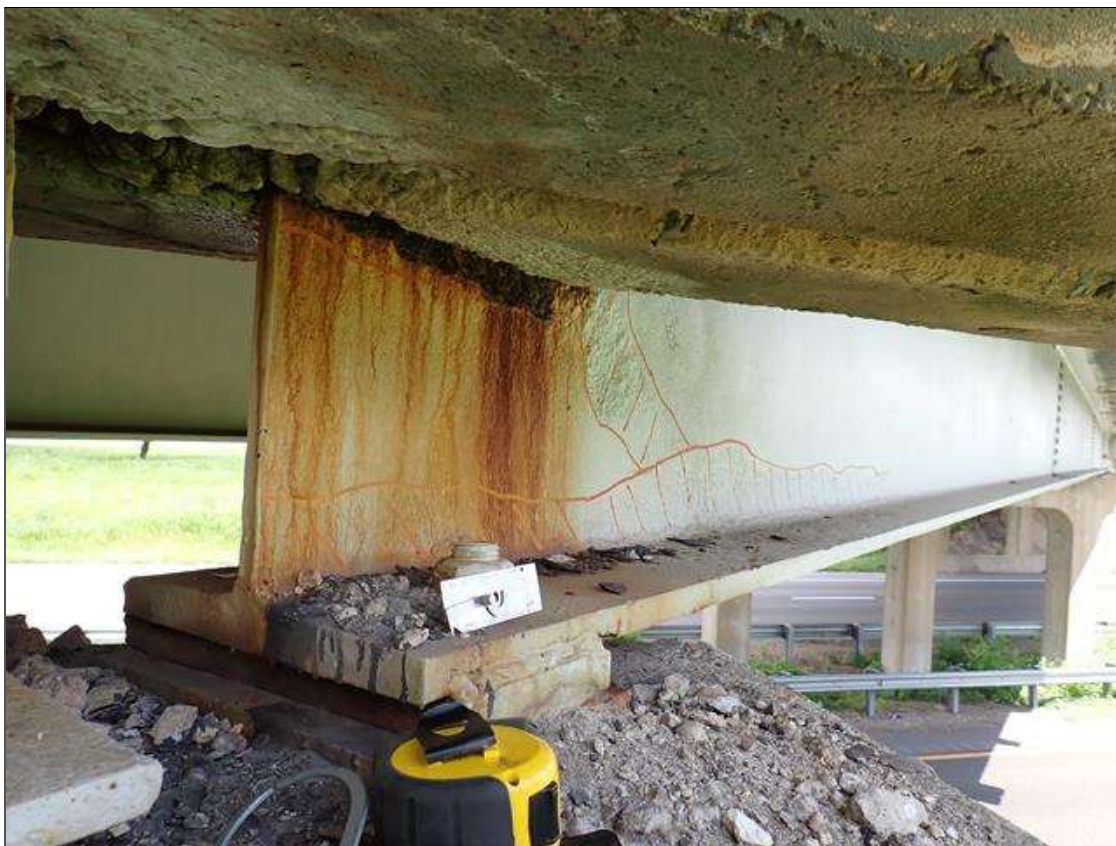
Span 2 Beam 4: (PAR) at bent 1, web adjacent to diaphragm, corrosion with section loss (3/16 inch average remaining x 18 inch x 5 inch); painted over section loss: lower web (5/16 inch average remaining x 5.5 feet x 4 inches); bottom flange, painted over pitting (up to 1/8 inch deep x 2.5 feet)
