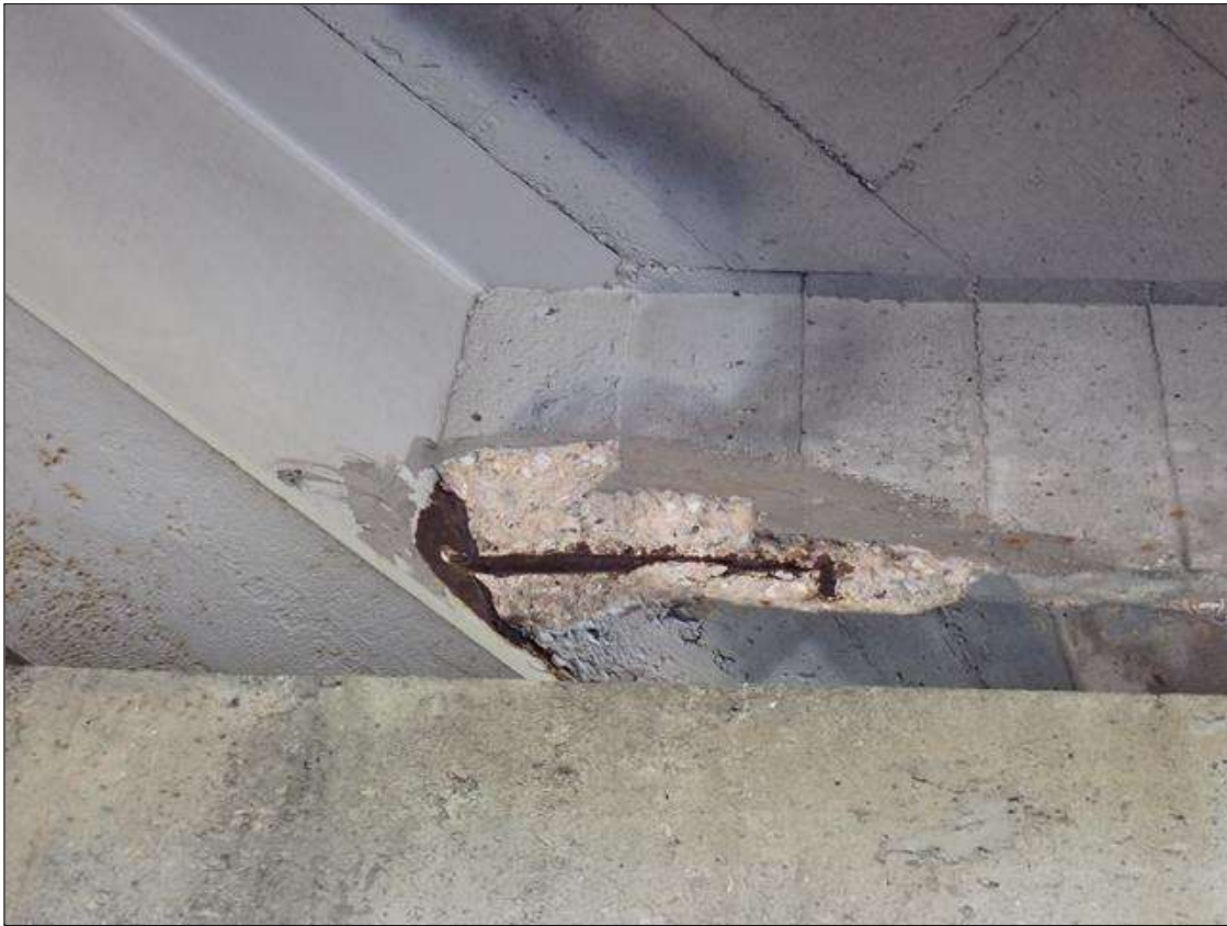
Span 2 Deck: at bents 1 and 2, end diaphragm, in all bays, spalls/delaminations/unsound patches (up to 2.5 feet x 10 inch x 3 inches deep) with exposed rusted rebar at random
