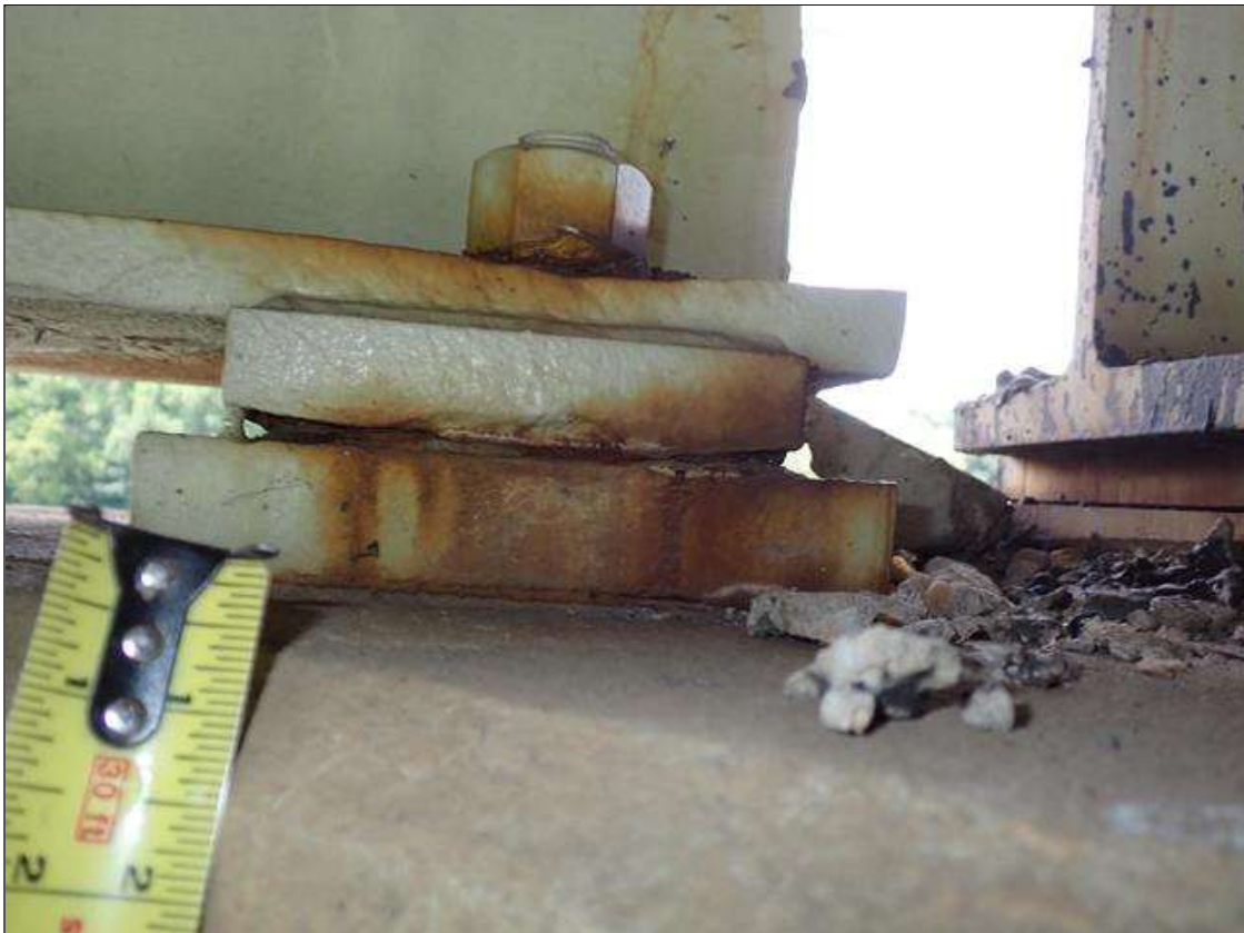
Span 2 Beam 1 - Far Bearing 1: FRECKLED RUST/PACK RUST ON ON THE BEARING PLATES.
