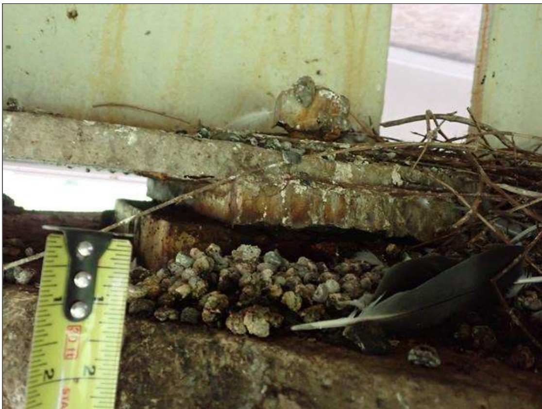
Span 4 Beam 2 - Near Bearing 2: SURFACE RUST/PACK RUST ON THE BEARING PLATES.
