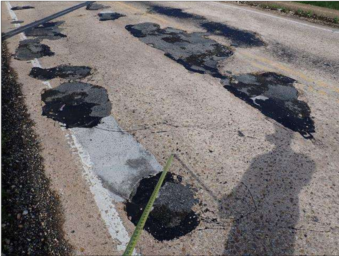
Span 3 Deck: (PAR) SPAN 3 TOP OF DECK HAS SCATTERED sound and unsound PATCHES [up to 8 feet x up to 4 feet x up to 1.5 inches deep] some with depressions; with adjacent spalls/delaminations (up to 1.5 foot diameter x 1.5 inches deep)
