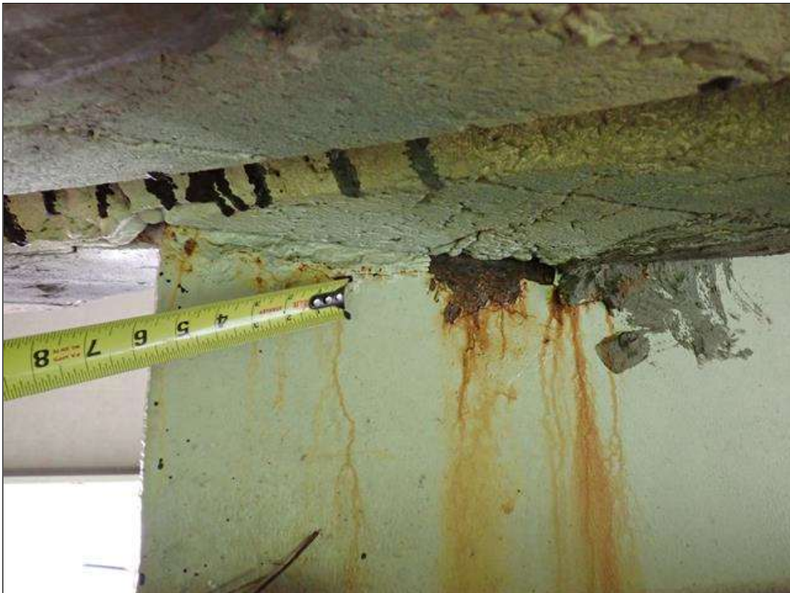
Span 3 Beam 2: (PAR) at bent 3, web adjacent to diaphragm, corrosion with section loss (3/8 inch average remaining x 14 inch x 2 inch)
