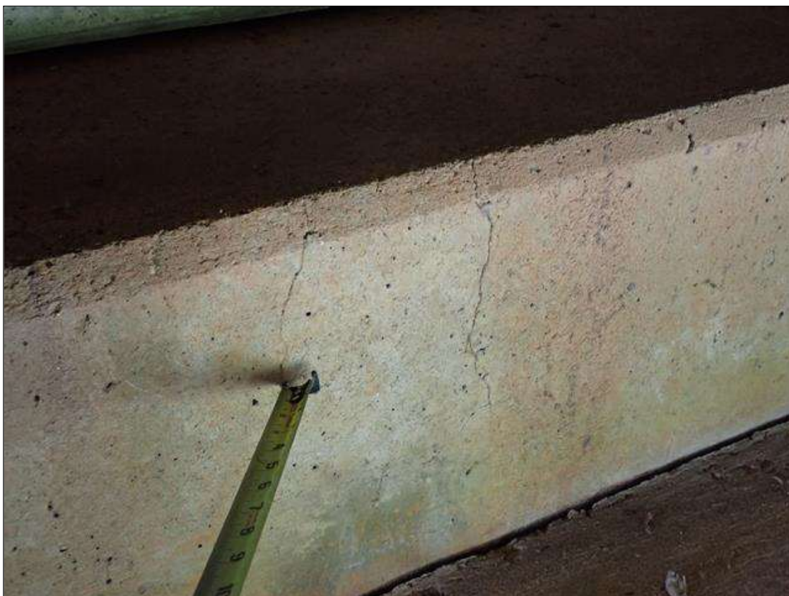
End Bent 2 Cap 1: along length, multiple vertical crack, up to full height x 1/64 inch, some extend across top face
