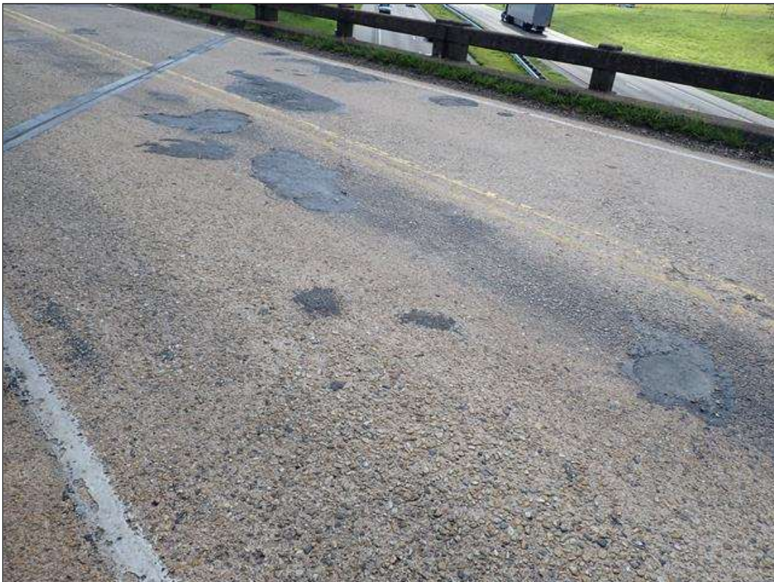
Span 3 Deck: 2023 previously repaired, previously noted as: in Southbound lane 10 feet from joint over bent 3, spall [up to 28 inch x up to 18 inch x up to 2 inch deep] with (1) exposed rusted reinforcing no section loss
