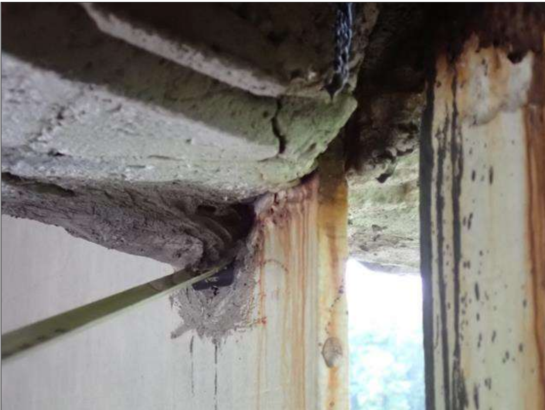
Span 3 Beam 1: (PAR) at bent 3, web adjacent to diaphragm, corrosion with section loss (5/16 inch average remaining x 1 foot x 3 inch)
