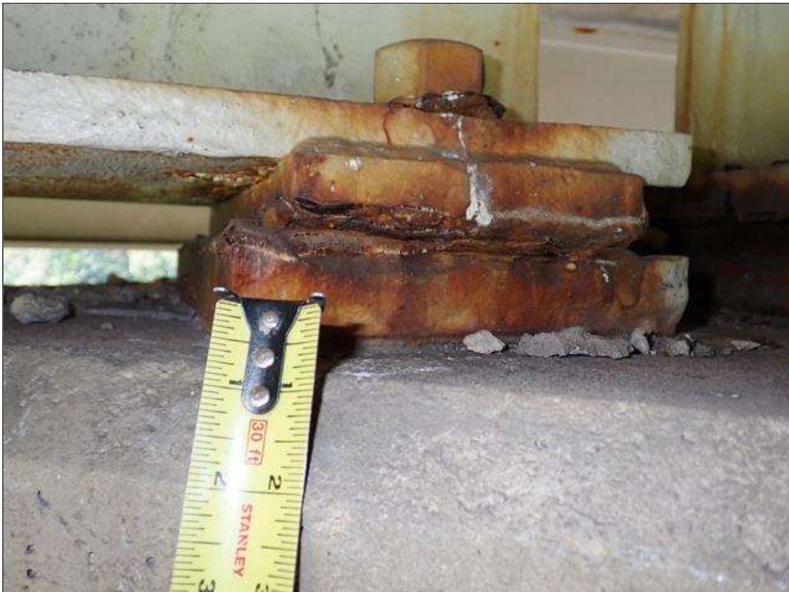
Span 2 Beam 2 - Far Bearing 2: painted over section loss (up to 1/8 inch deep) with corrosion reinitiated; pack rust
