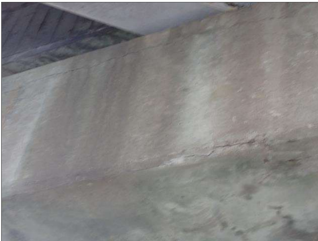
Bent 3 Cap 1: south face, upper and lower edges, longitudinal cracks (up to 1/8 inch x full length) with adjacent delaminations (up to 8 feet x 8 inch)
