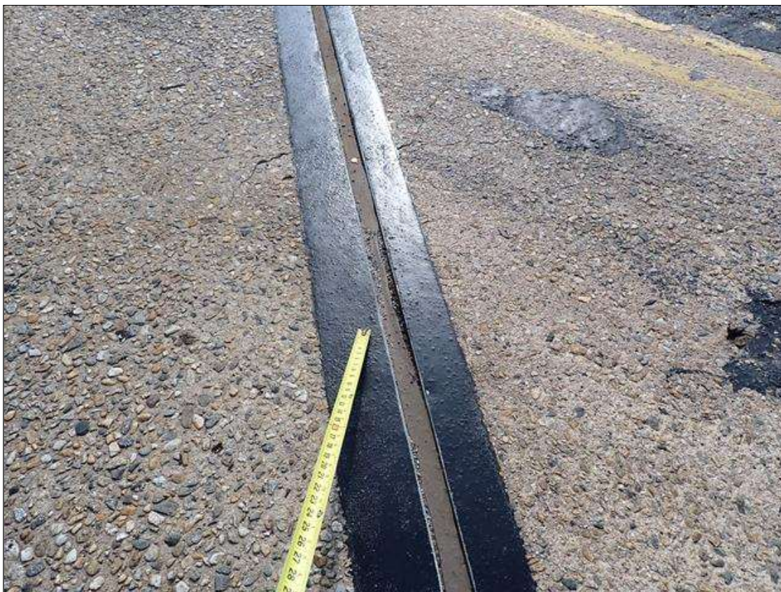
Span 4 Bent 3 Joint: along the length of the joint, areas of adhesion loss at random
