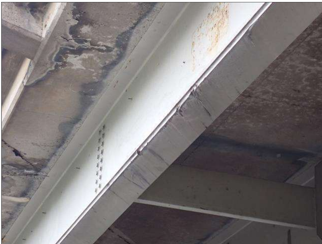
Span 3 Beam 4: (PAR) cover plate over right travel lane and shoulder, impact scrapes with gouges (approximately 1/2 inch deep)
