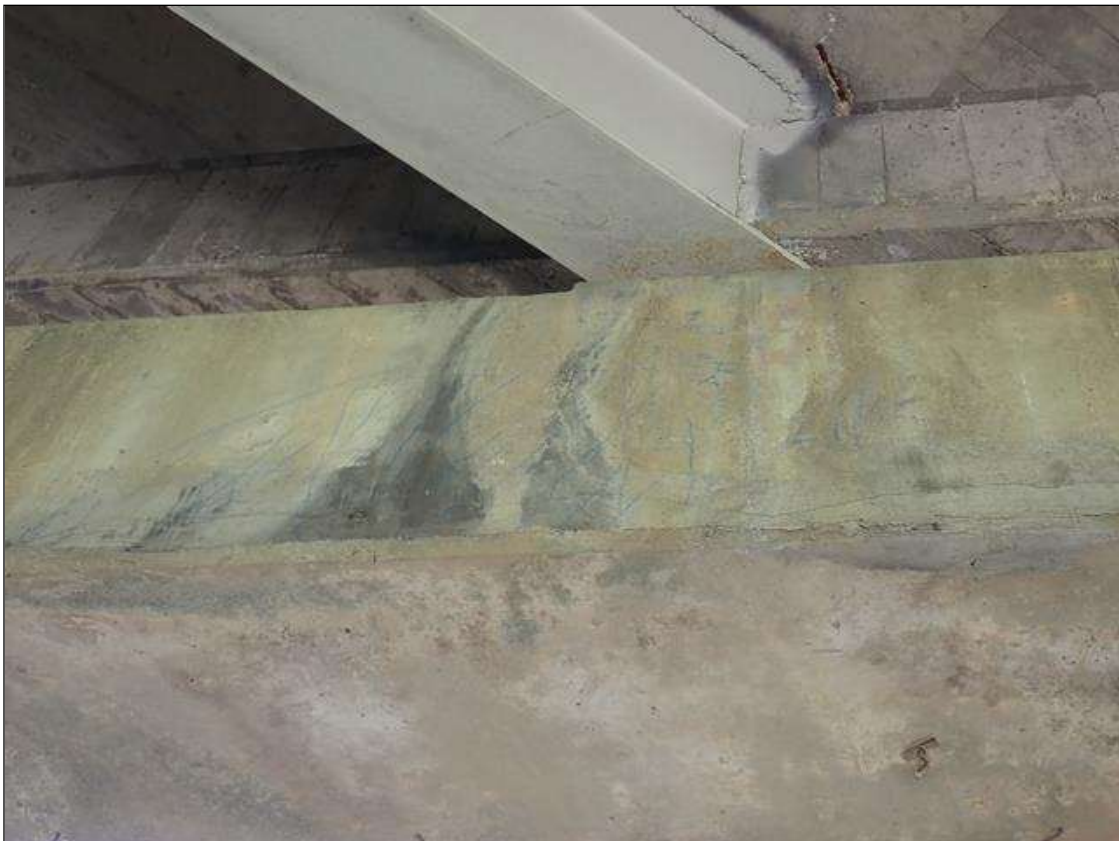
Bent 2 Cap 1: south and north faces of cap, multiple delaminations/spalls (up to 8 feet x 2 feet x 1.5 inch deep), some with exposed rusted rebar and associated cracks (up to 1/8 inch wide)
