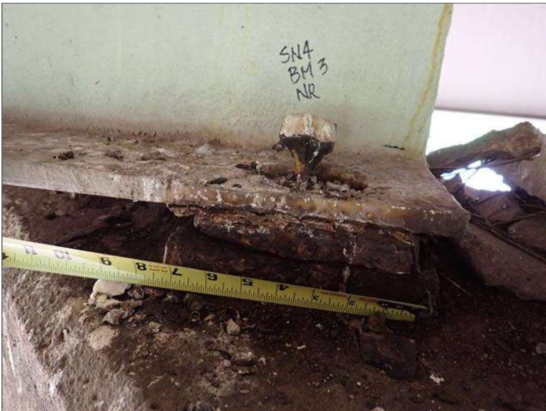
Span 4 Beam 3 - Near Bearing 3: (PAR) west side of bearing, between sole and beam bottom flange, broken weld
