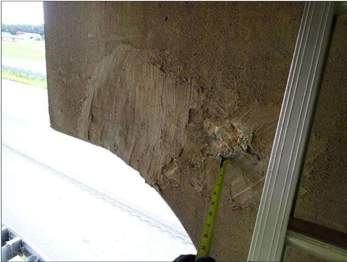
Bent 3 Cap 1: north face of cap, bay 3 to right end, delamination/unsound patches/spalls (up to 7.5 feet x 1 foot x 1/2 inch deep) with associated cracks (up to 1/16 inch)
