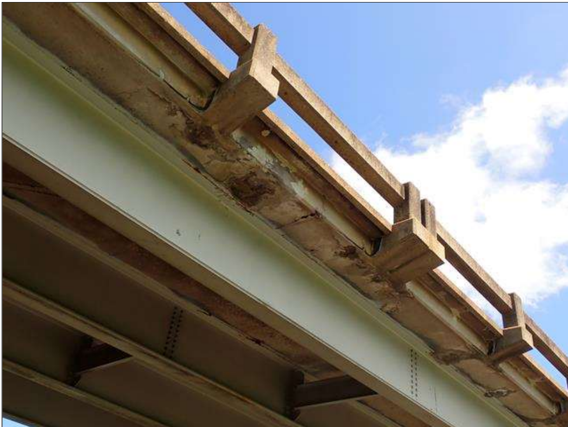
Span 2 Deck: (PAR) SPAN 2 BOTTOM OF DECK EAST OVER HANG HAS SCATTERED unsound PATCH AREAS THROUGH OUT with associated delaminations [up to 30 inch diameter] over traffic
