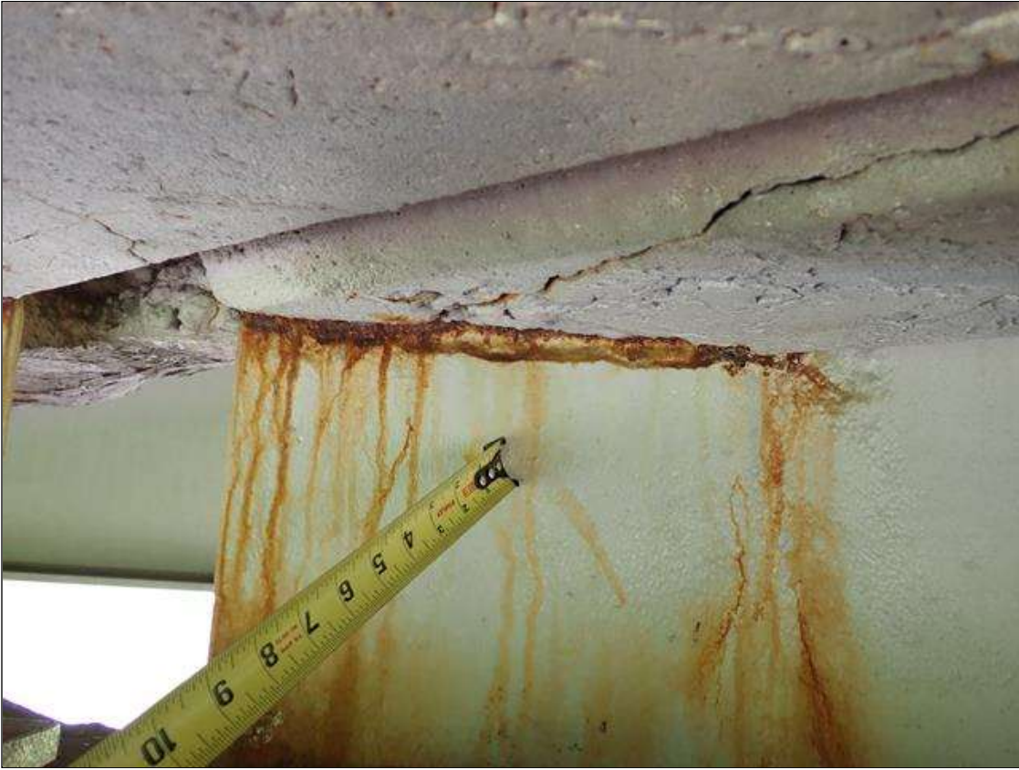
Span 3 Beam 3: (PAR) at bent 2, web adjacent to diaphragm, painted over section loss (1/4 inch average remaining x 14 inch x 3 inch) with adjacent painted over pitting (up to 1/8 inch deep) with corrosion reinitiated
