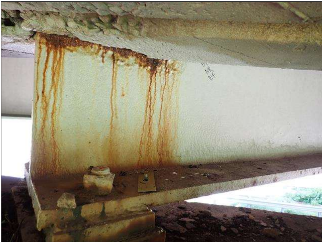
Span 2 Beam 3: (PAR) at bent 1, painted over section loss: web adjacent to diameter (5/16 inch average remaining x 14 inch x 3 inch); lower web (3/8 inch average remaining x 3 feet x 3 inches) with corrosion reinitiated
