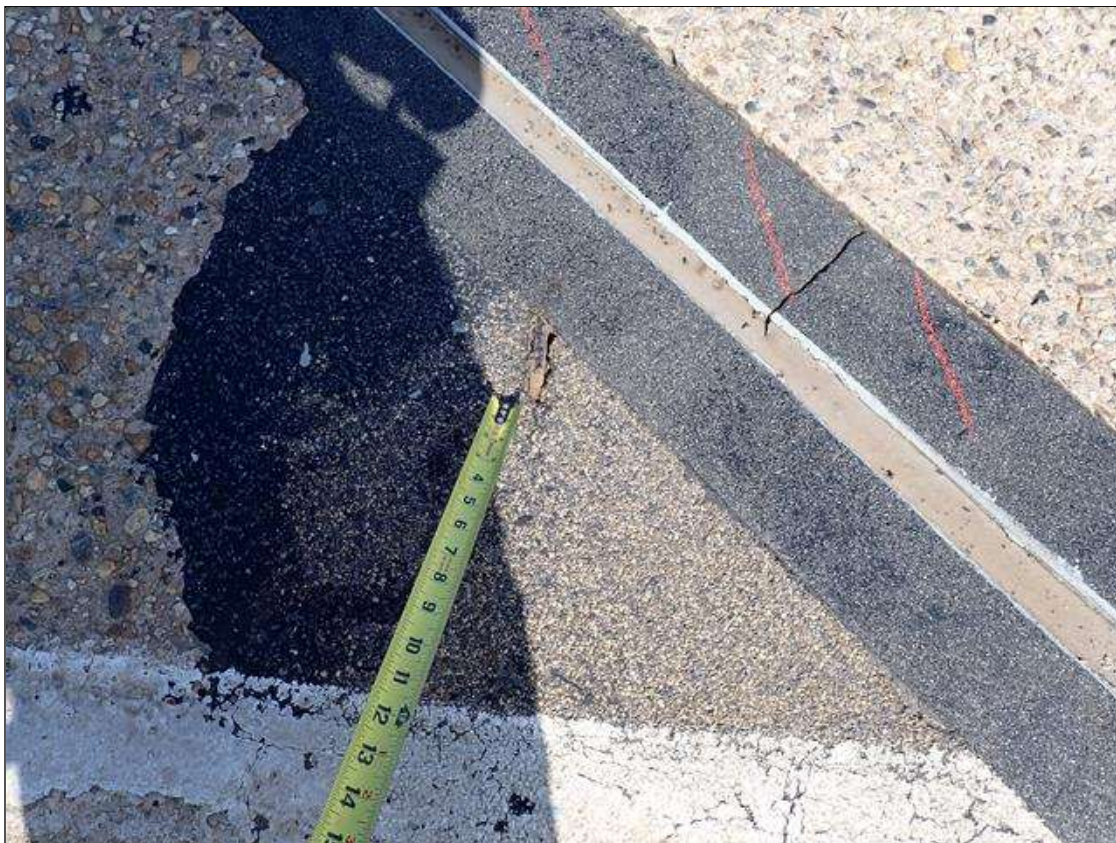
Span 1 Deck: (PAR) northbound lane, adjacent to bent 1 and right shoulder, shallow rebar; rebar has less than 5 percent section loss
