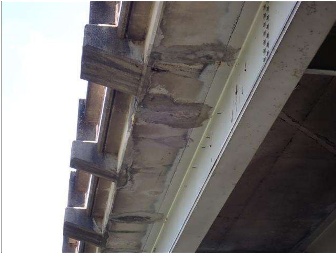
Span 2 Deck: (PAR) SPAN 2 BOTTOM OF DECK WEST OVERHANG HAS SCATTERED unsound PATCHED AREAS THROUGH OUT SPAN with some associated delaminations [up to 30 inch diameter] over traffic
