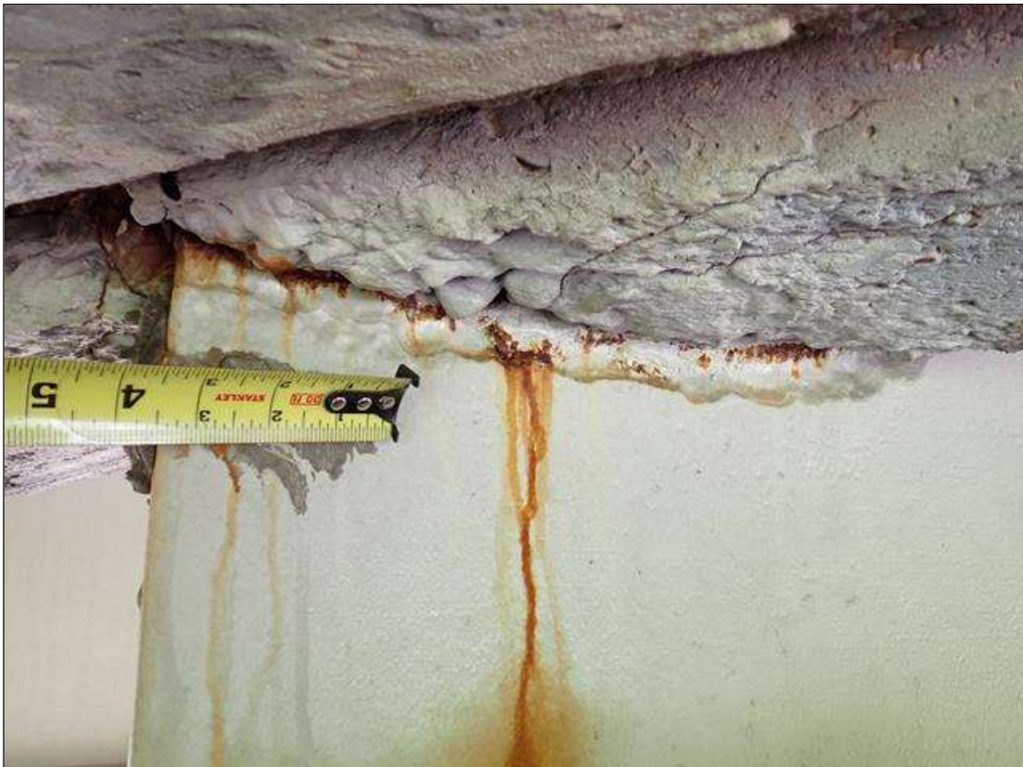
Span 3 Beam 2: (PAR) at bent 2, web adjacent to diaphragm, painted over section loss (1/4 inch average remaining x 15 inch x 2 inch) with corrosion reinitiated
