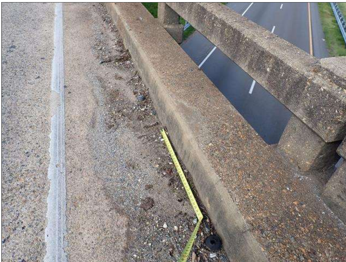
Span 2 Left Bridge Rail: face of curb, near bent 1, patched area (34 feet x 9 inch) with cracks (up to 1/32 inch)
