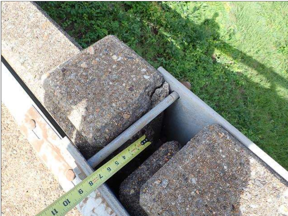
Span 1 Left Bridge Rail: at Southwest guardrail attachment in top of rail post, spall [10 inches x 10 inches x 1.5 inches deep] no exposed reinforcing
