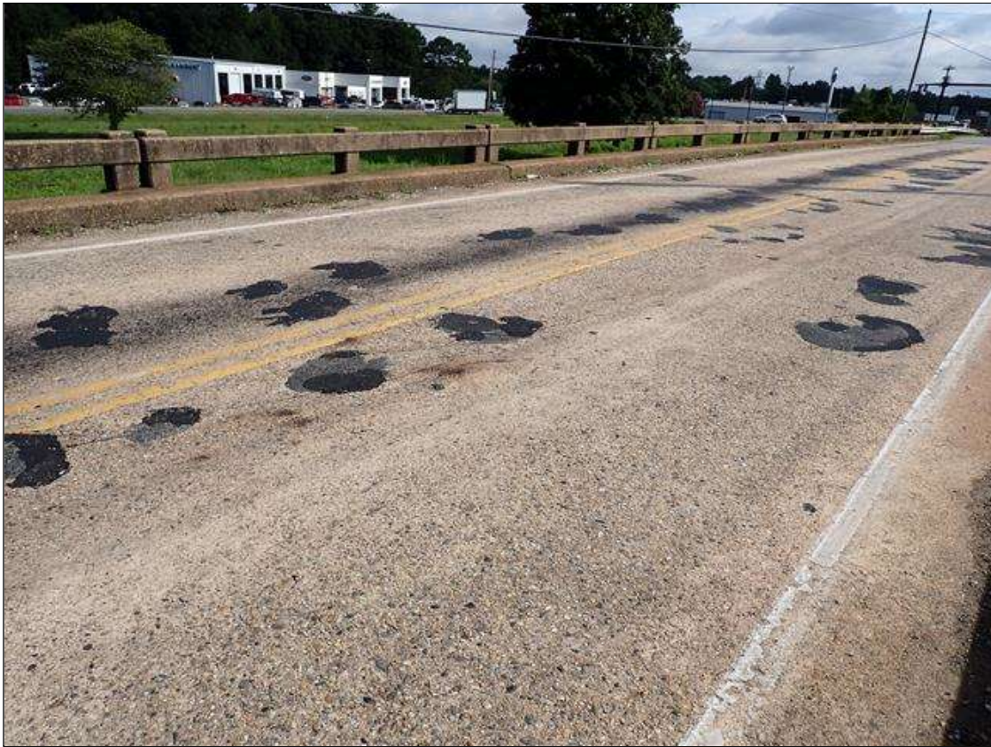
Span 2 Deck: 2023 previously repaired, previously noted as: in Northbound lane near midspan, (2) spalls [up to 16 inch x 21 inch x up to 2 inch deep] with (2) exposed rusted reinforcing no section loss
