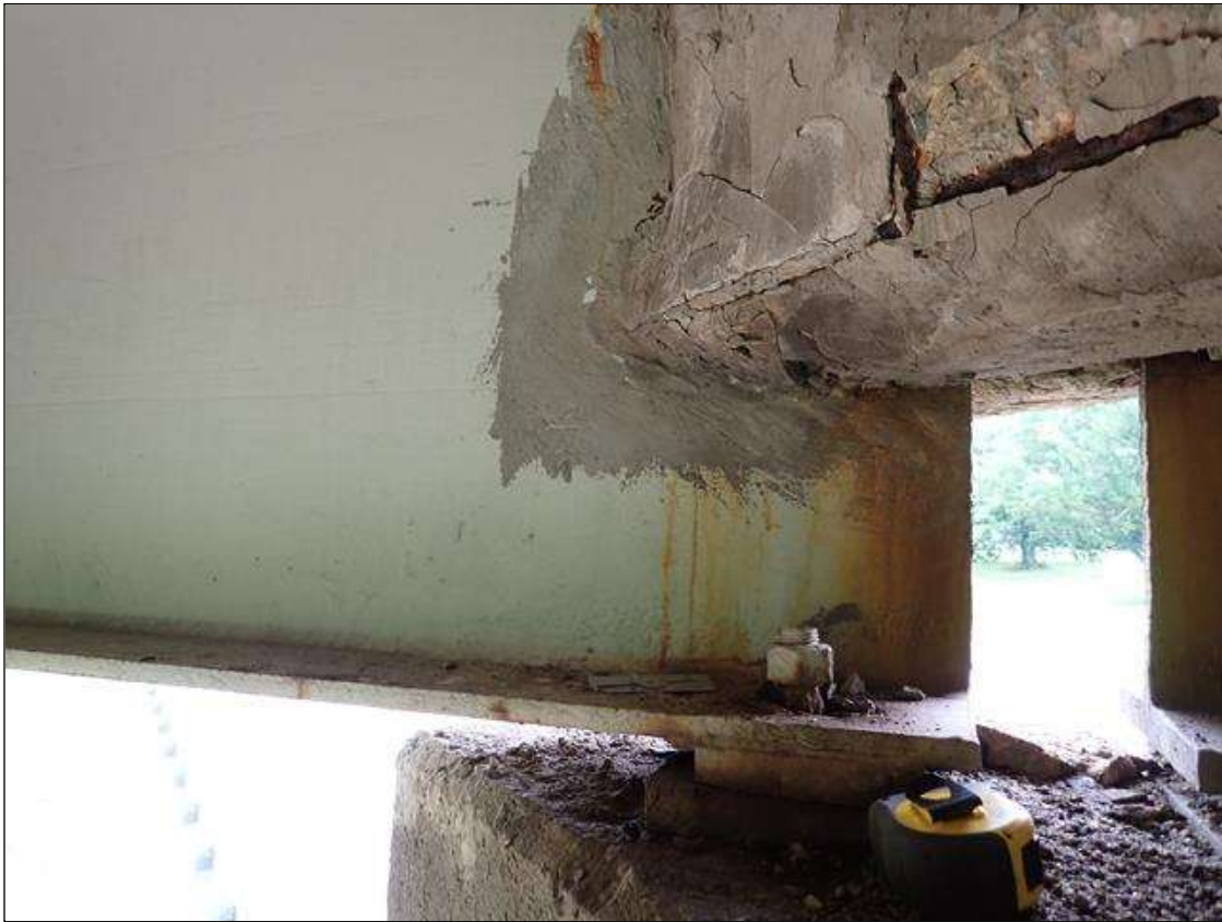
Span 4 Beam 4: (PAR) at bent 3, painted over section loss: web adjacent to diaphragm (5/16 inch average remaining x 9 inch x 2 inch); lower web (7/16 inch average remaining x 1 foot x 3 inch); bottom flange (0.75 inch average remaining x 6 inches) with corrosion reinitiated
