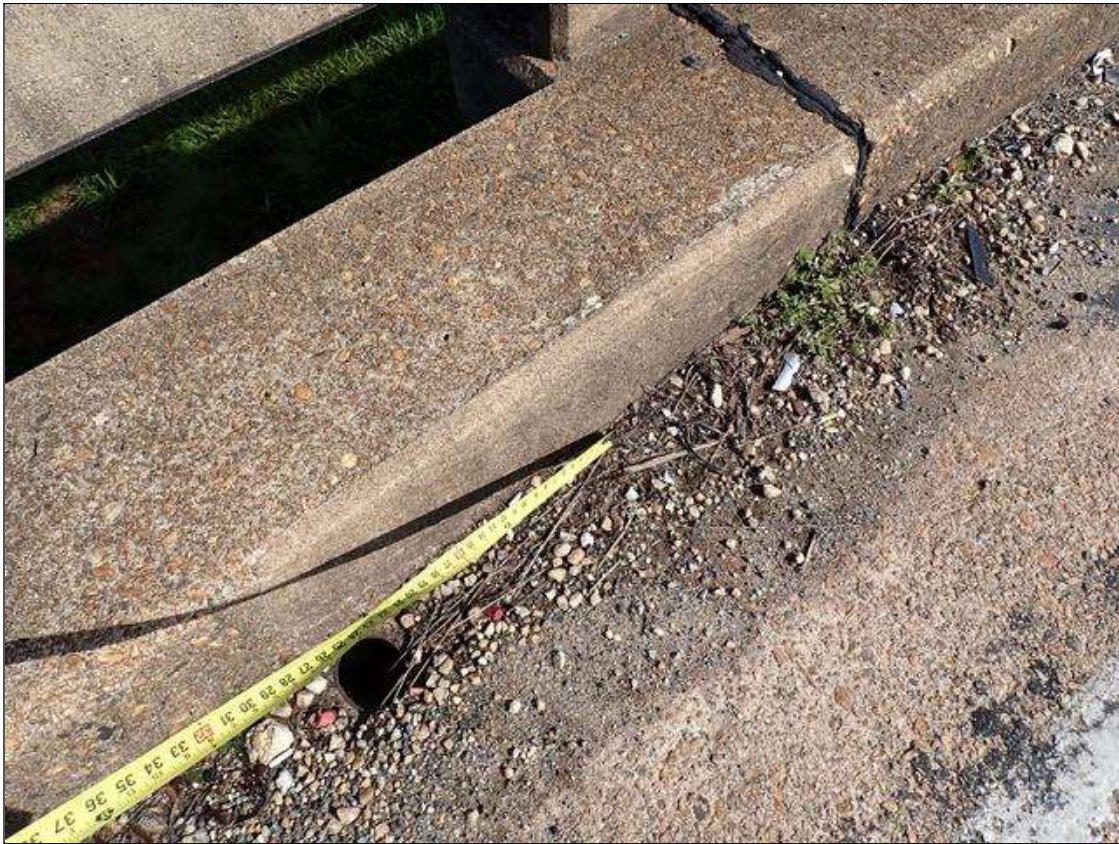
Span 3 Left Bridge Rail: adjacent to joint over bent 3, sound patched area [4 feet x 11 inches] with associated hairline map cracking
