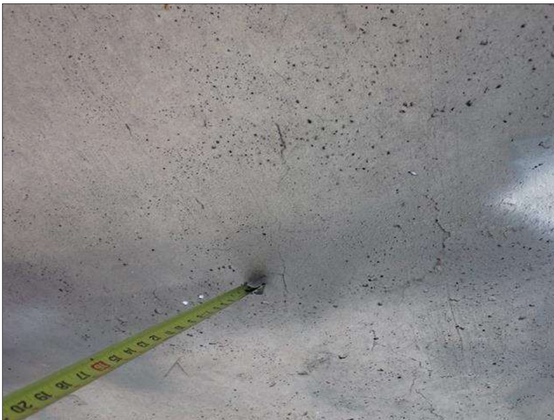
Span 4 Deck: throughout underside of deck, areas of map cracks (hairline) at random
