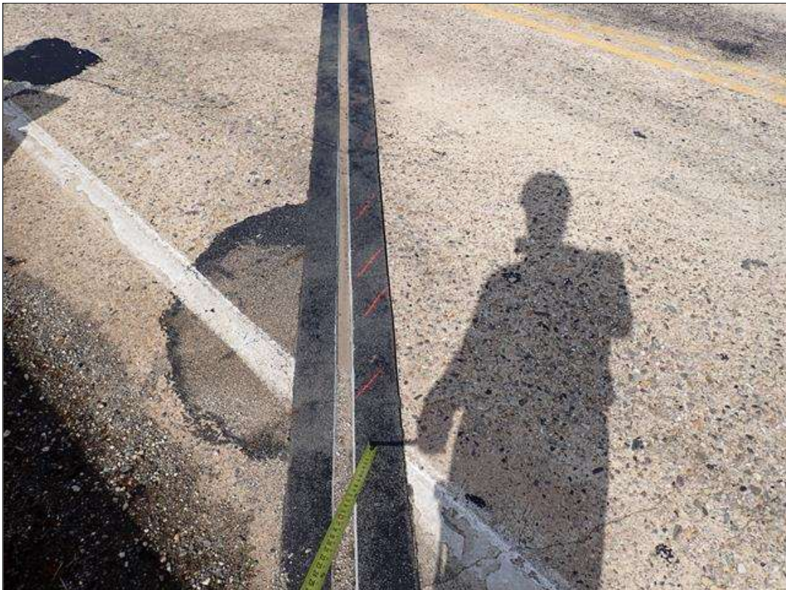
Span 2 Bent 1 Joint: (PAR) spans 1 and 2 header, in both travel lanes, delaminations (up to 12.5 feet x 6 inches) with cracks (up to 1/8 inch) and separated from adjacent deck (up to 1/2 inch)
