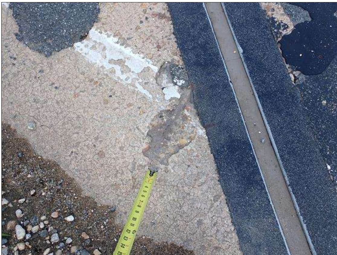
Span 2 Deck: (PAR) right shoulder, at bent 2, spall (1 foot x 6 inch x 1 inch deep) with exposed rusted rebar
