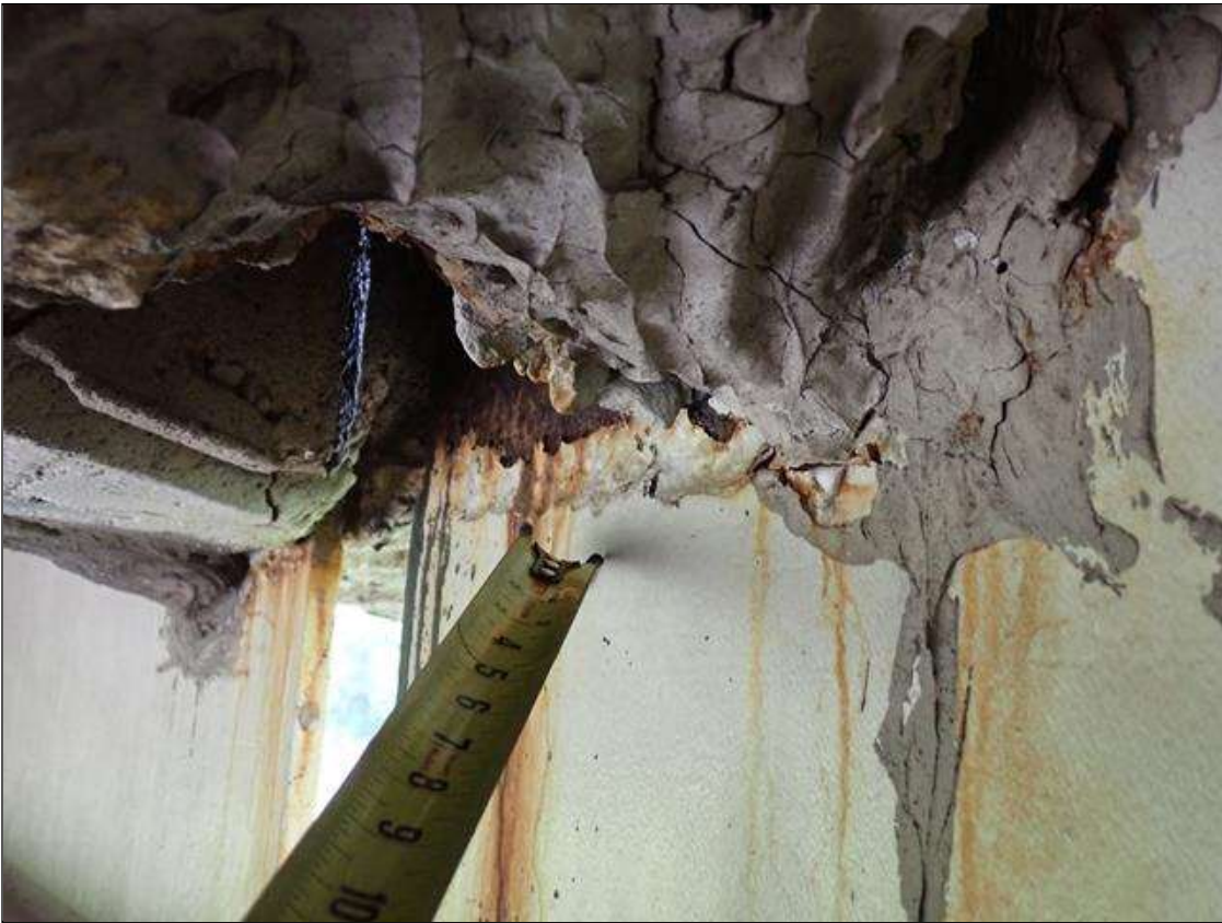
Span 4 Beam 1: (PAR) at bent 3, web adjacent to diaphragm, corrosion with section loss (1/4 inch average remaining x 15 inch x 4 inch)
