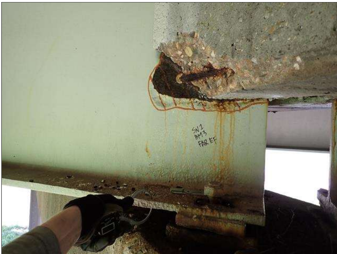
Span 1 Beam 3: (PAR) at bent 1, web adjacent to diaphragm, corrosion with section loss (1/4 inch average remaining x 12 inch x 6 inch); painted over section loss: lower web (5/16 inch average remaining x 16 inch x 3 inch), bottom flange (0.63 inch average remaining x 15 inches)
