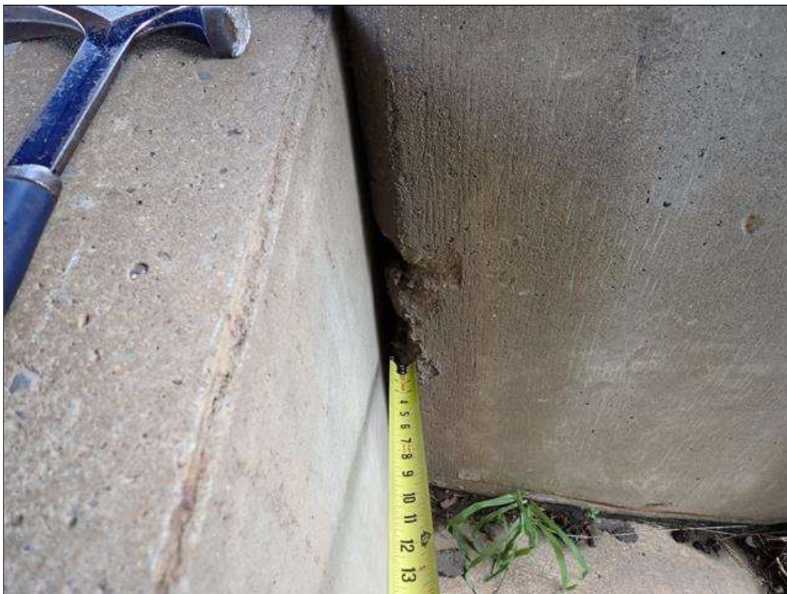
Bent 1 Pile 3: northwest corner, near ground, spall (10 inch x 4 inch x 1.5 inch deep)
