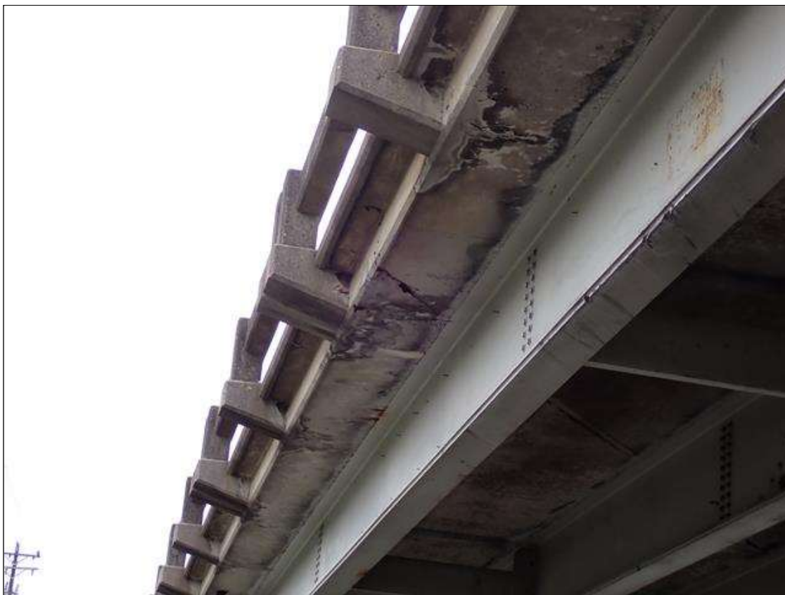
Span 3 Deck: [PAR] SPAN 3 BOTTOM OF DECK RIGHT OVER HANG HAS SCATTERED UNSOUND PATCHED AREAS THROUGH OUT THE SPAN WITH ASSOCIATED DELAMINATIONS [UP TO 18 INCH X UP TO 3 FEET] OVER TRAFFIC
