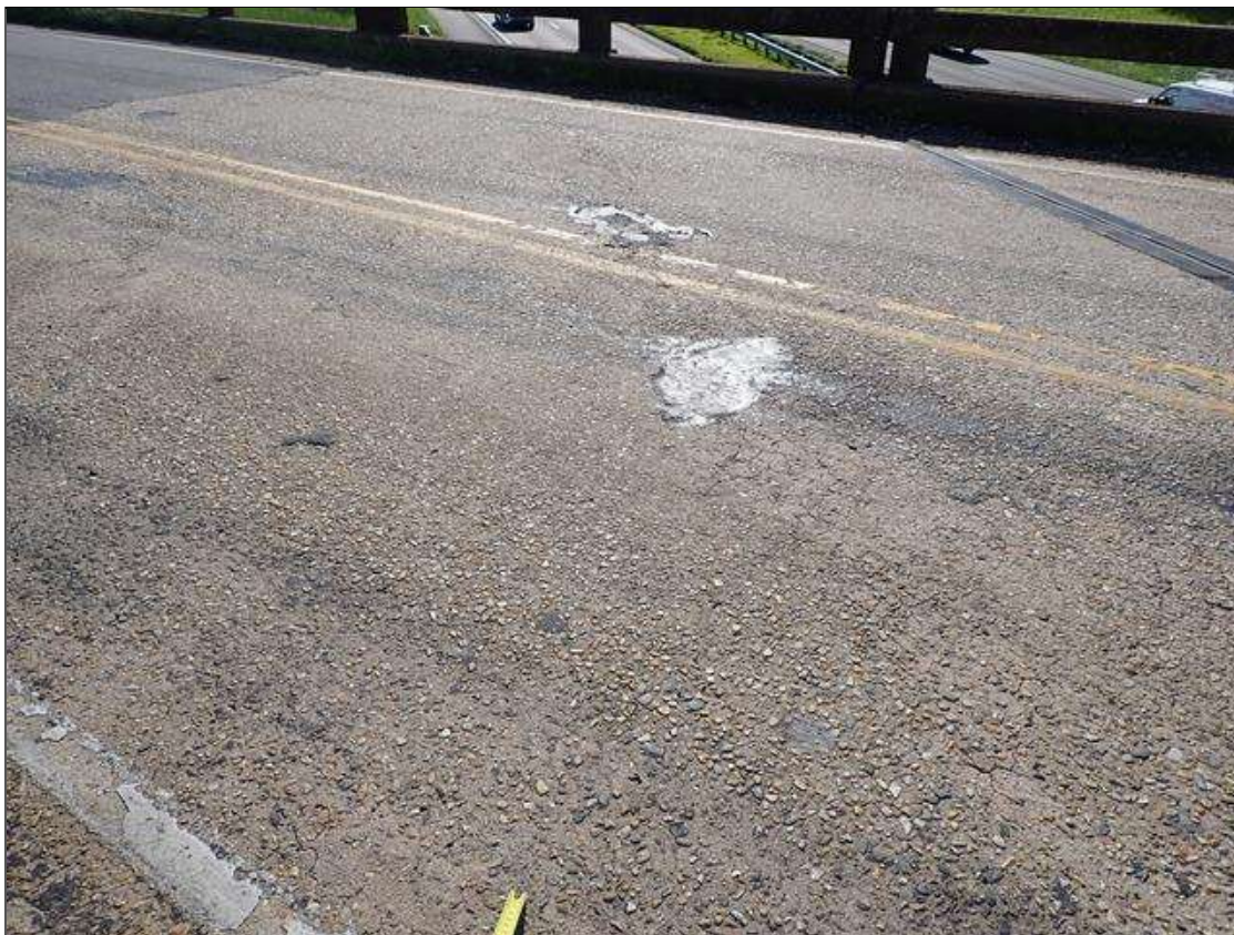
Span 4 Deck: SPAN 4 TOP OF DECK HAS SCATTERED sound and unsound PATCHES [up to 2 foot diameter x up to 1/2 inch deep]
