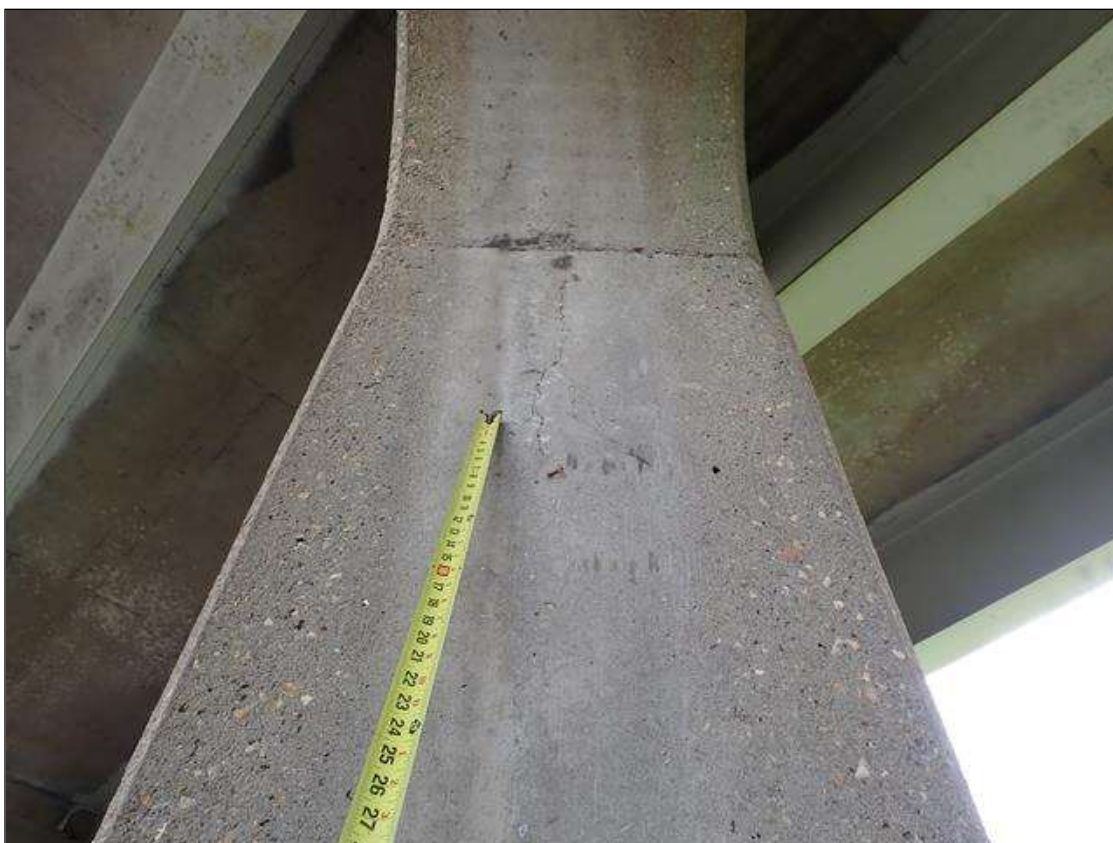
Bent 1 Pile 2: UP TO 3 FOOT X 1/32 VERTICAL CRACK WEST FACE AT BOTTOM OF CAP
