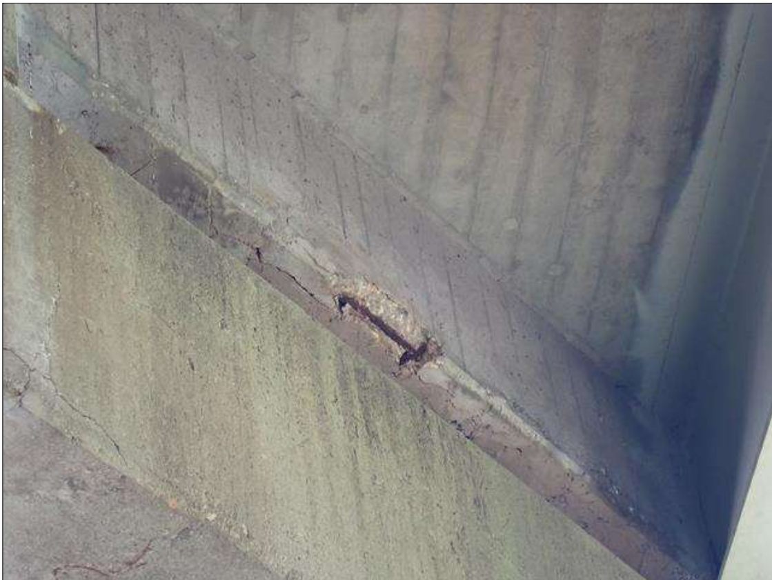
Span 1 Deck: at bent 1, bay 2 end diaphragm, spall/delamination (4 feet x 6 inch x 2 inch deep)
