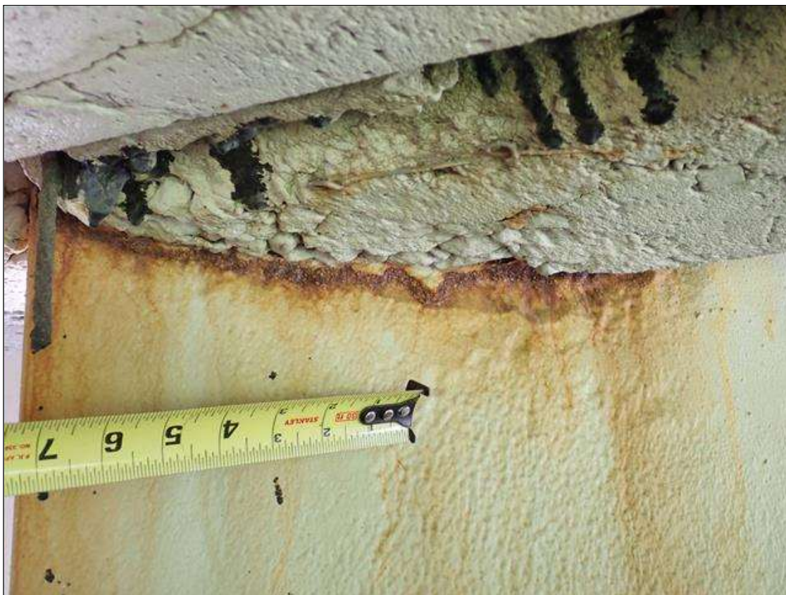
Span 2 Beam 2: (PAR) near end web at diaphragm, arrested metal loss/pitting, 12 inch long x up to 2 inch high x average remaining 5/16 inch with reactivated surface corrosion
