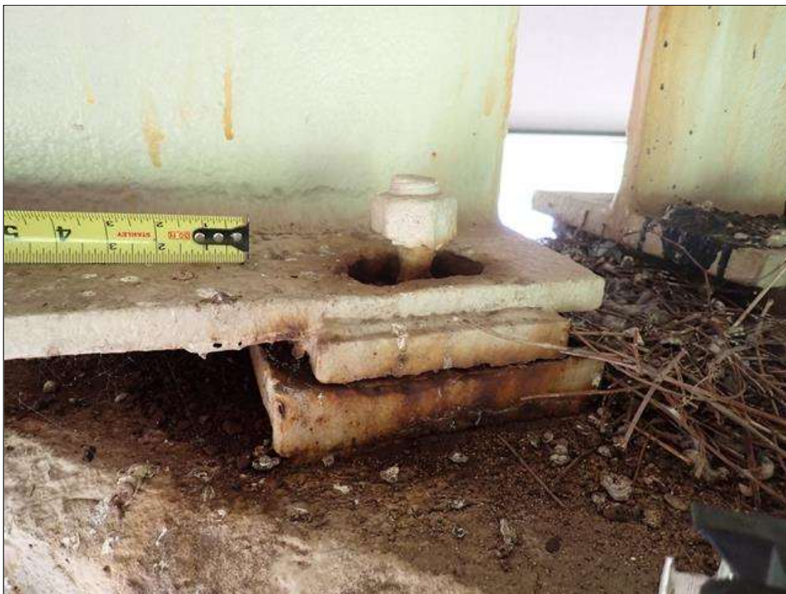
Span 1 Beam 2 - Far Bearing 2: (PAR) rust scale; right anchor bolt, painted over section loss (50 percent average remaining)
