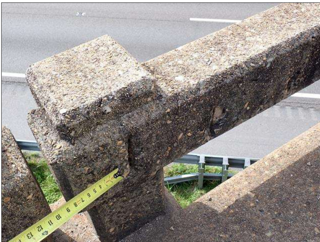
Span 4 Right Bridge Rail: rail, near midspan, spalls (up to 6 inch x 3 inch x 3/4 inch deep) with exposed rusted rebar
