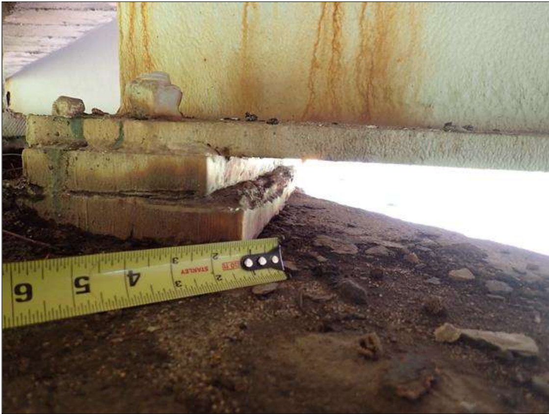
Span 2 Beam 3 - Near Bearing 3: painted over section loss (up to 1/4 inch deep); pack rust
