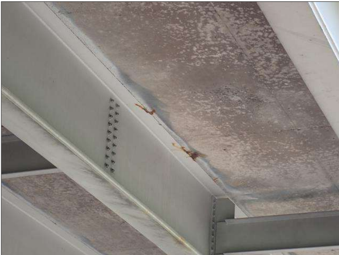
Span 2 Deck: (PAR) bay 3, adjacent to beam 3, near 2nd intermediate diaphragm, rust stains
