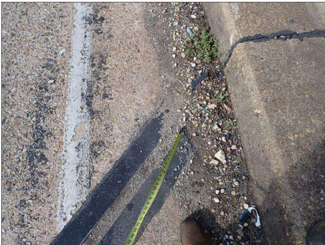
Span 4 Bent 3 Joint: both shoulders, debris accumulation
