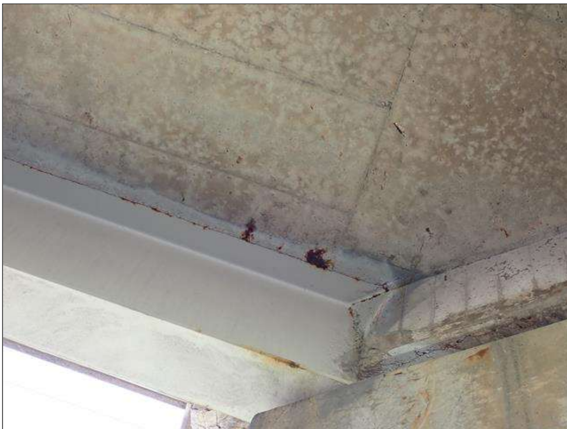
Span 3 Deck: (PAR) underside of bays 1 and 3, adjacent to beams, areas of rust stains at random
