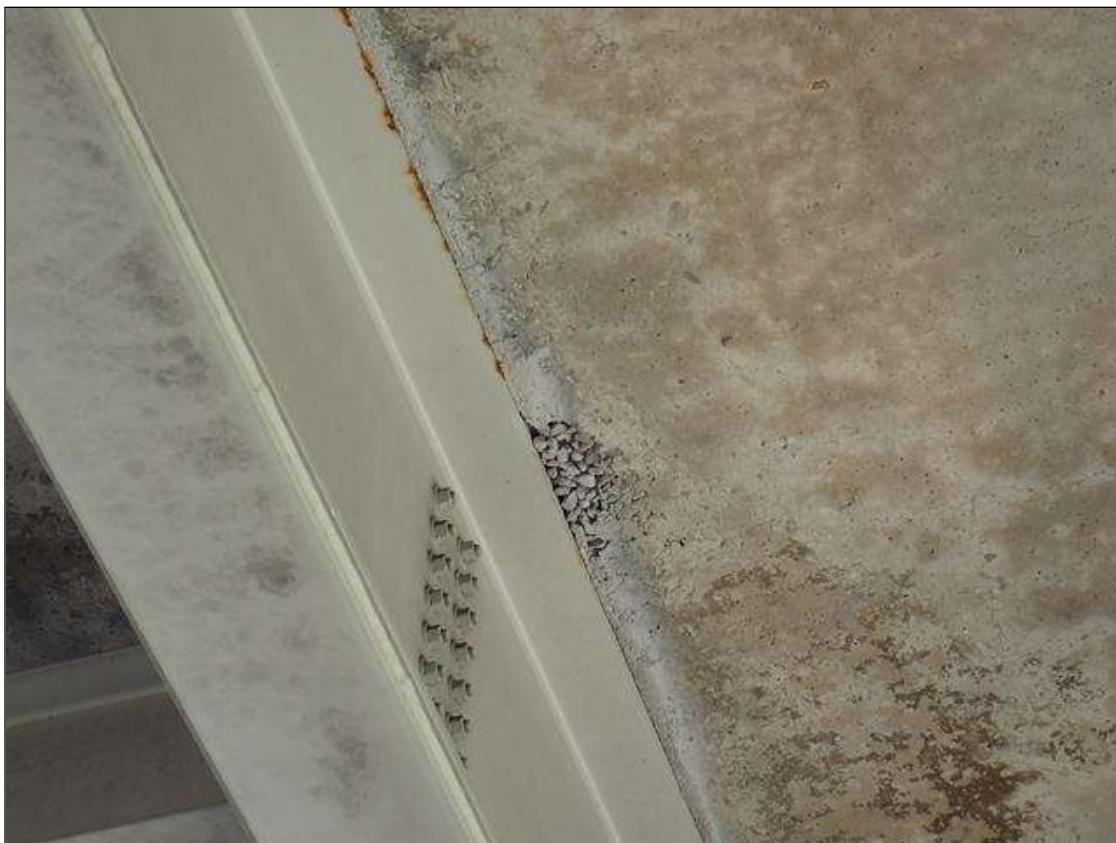
Span 3 Deck: underside of bays 2 and 3, near half of span, areas of poor consolidation (up to 3.5 feet x 15 inch x 1 inch deep)
