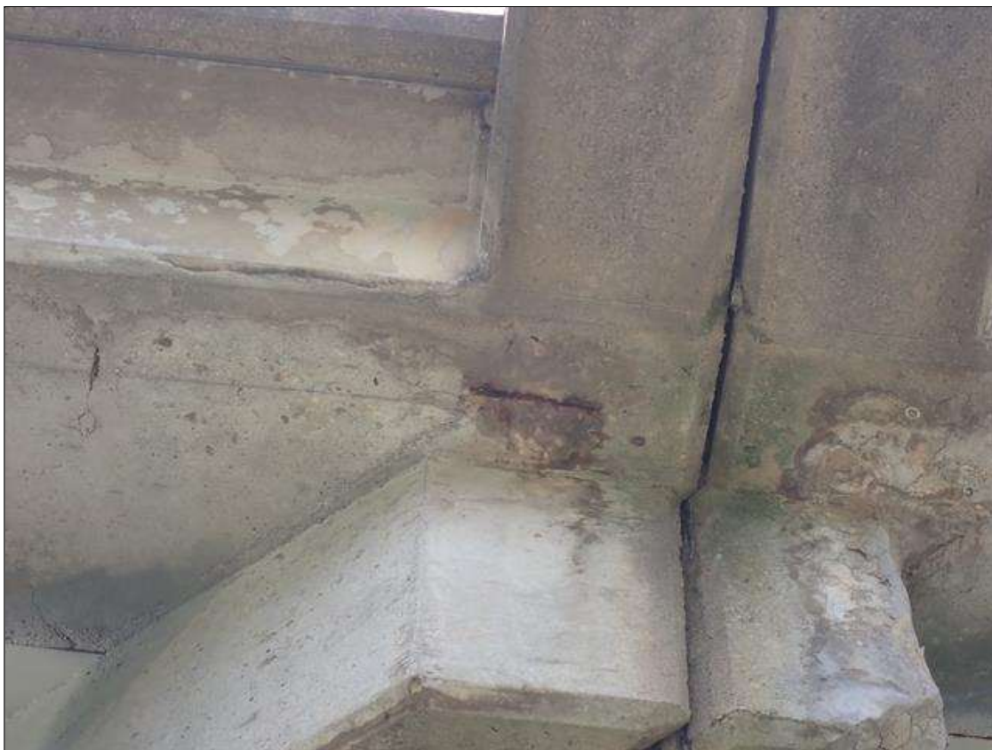
Span 2 Deck: (PAR) on right overhang at bent 2, spall [7 inch x 1 inch x 1/2 inch deep] with exposed rusted reinforcing
