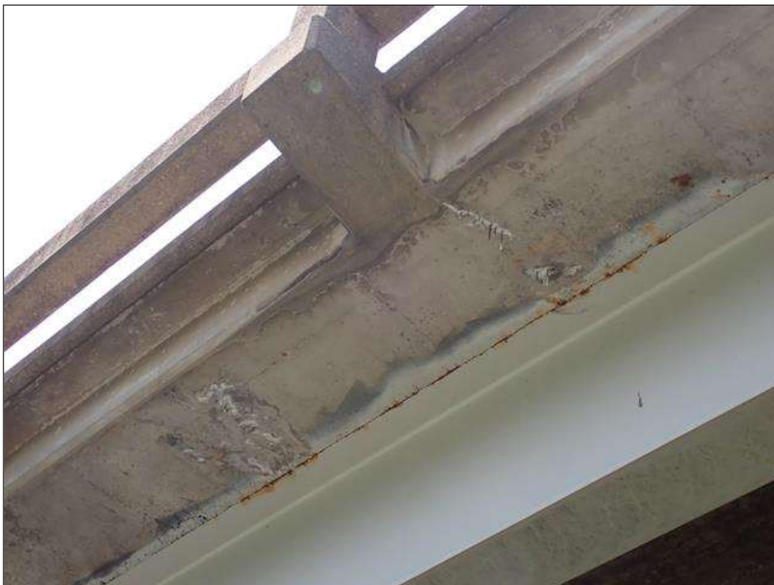
Span 2 Deck: (PAR) underside of right overhang near bent 2, multiple transverse cracks [up to 1/64 inch] with some efflorescence buildup
