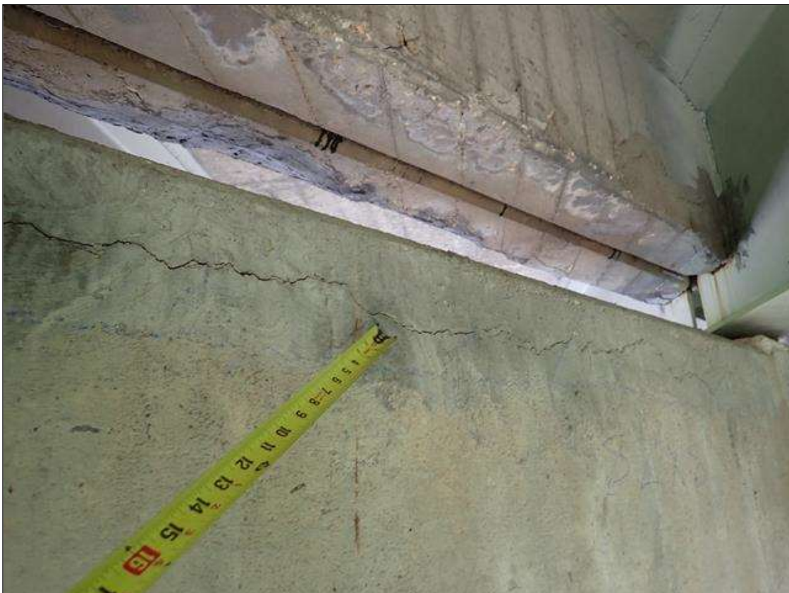
Bent 3 Cap 1: north face of cap, bay 3 to right end, delamination/unsound patches/spalls (up to 7.5 feet x 1 foot x 1/2 inch deep) with associated cracks (up to 1/16 inch)
