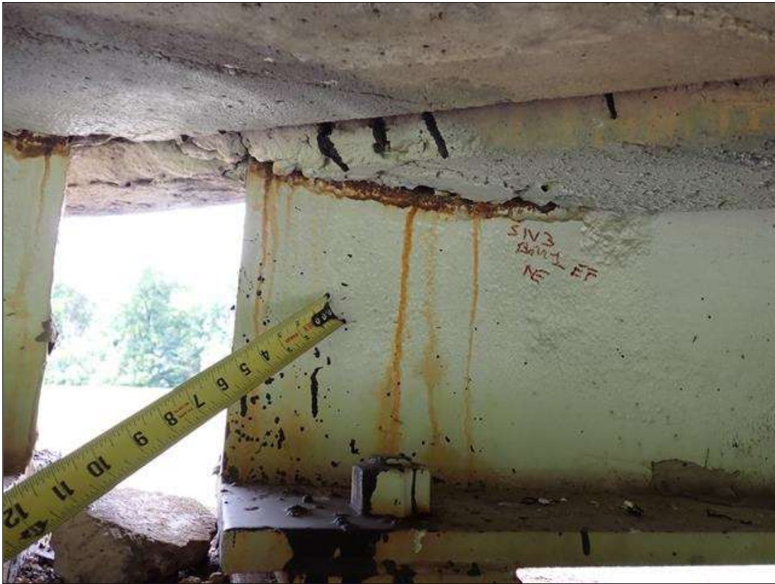
Span 3 Beam 1: (PAR) at bent 2, web adjacent to diaphragm, painted over section loss (5/16 inch average remaining x 14 inch x 4 inch); lower web, painted over pitting (up to 1/8 inch deep x 17 inch x 6 inch) with corrosion reinitiated
