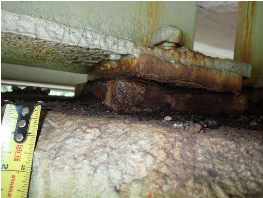
Span 1 Beam 3 - Far Bearing 3: rust scale/pack rust
