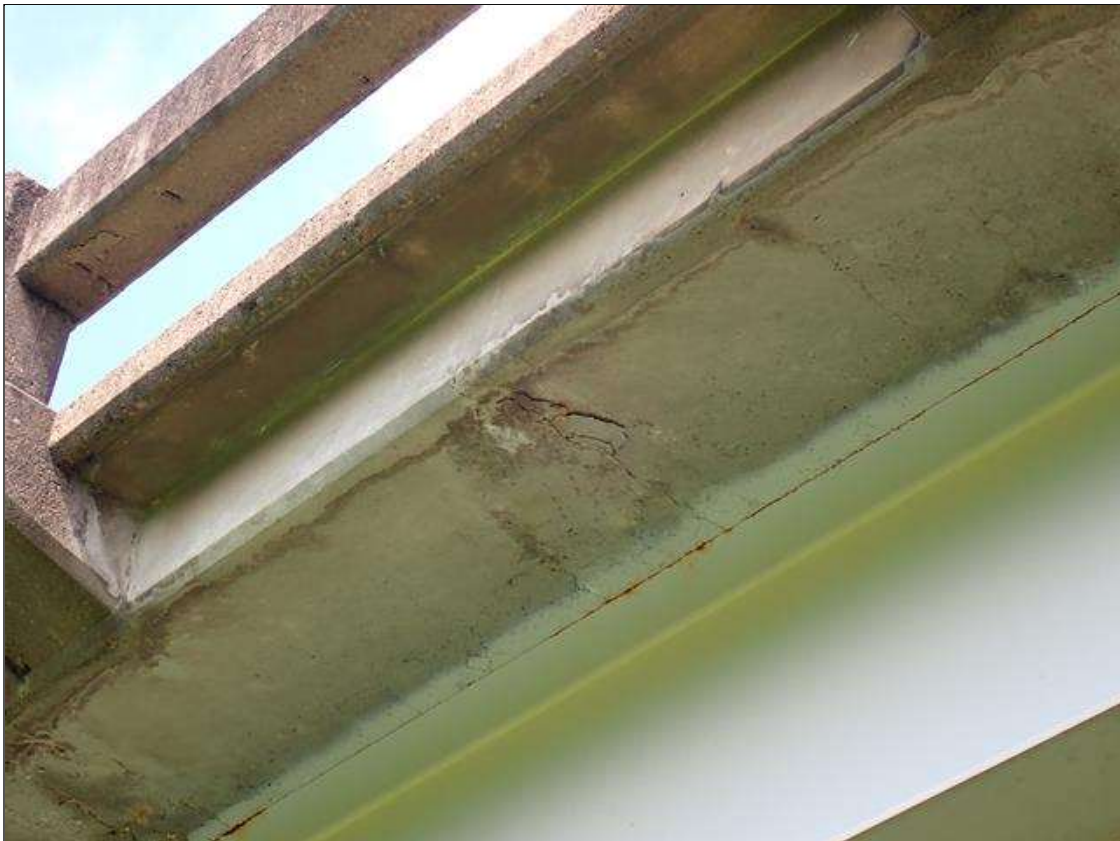
Span 1 Deck: SPAN 1 BOTTOM OF DECK IN RIGHT OVER HANG HAS SCATTERED unsound PATCHED AREAS with associated delaminations [up to 12 inch diameter]
