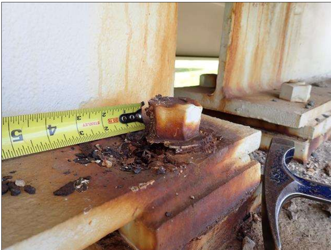
Span 2 Beam 4 - Far Bearing 4: right anchor bolt nut, painted over section loss up to 10 percent with corrosion reinitiated
