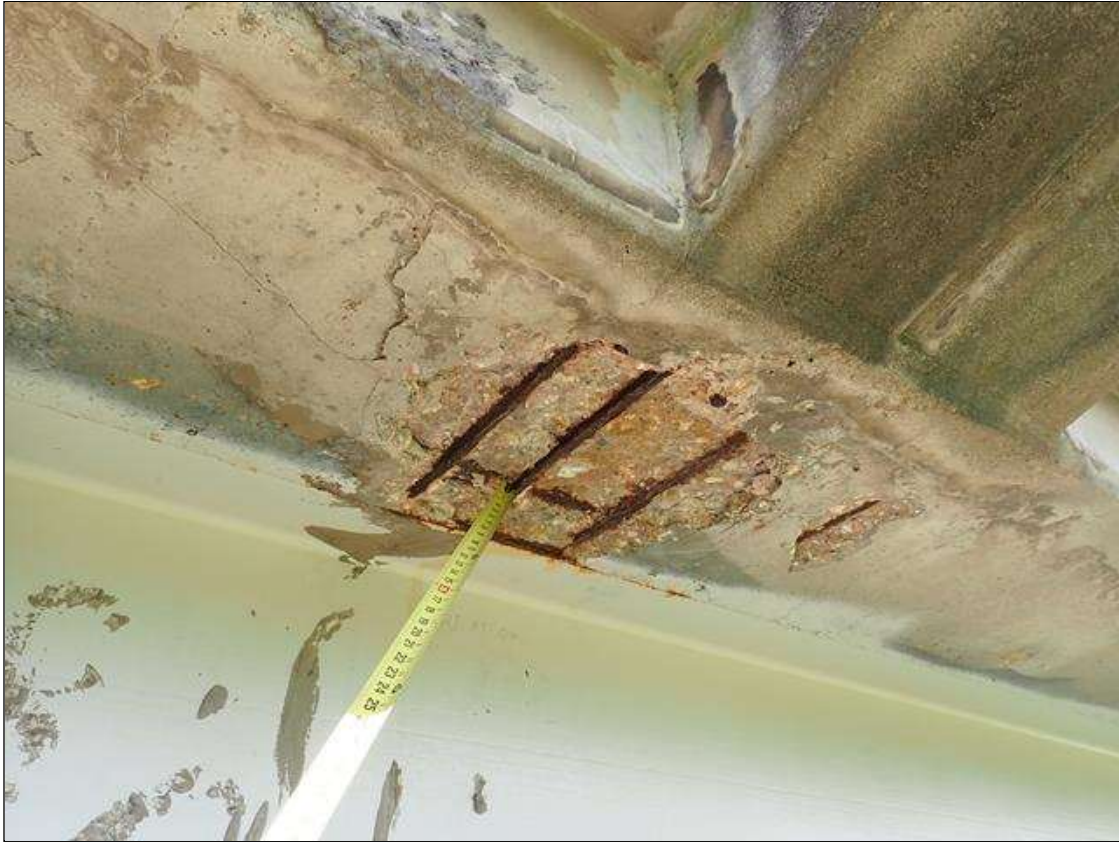
Span 1 Deck: (PAR) underside of deck on right overhang 20 feet from end bent 1, spall [2 feet x 3 feet x up to 2.5 inches deep] with multiple exposed rusted reinforcing [section loss up to 10 percent]
