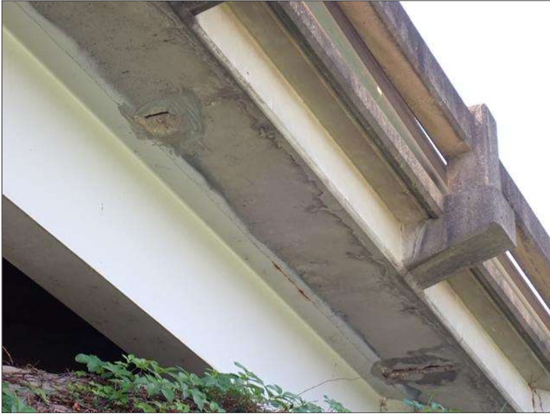
Span 1 Deck: (PAR) underside of deck on left overhang, multiple failed patches/spalls [up to 18 inches x 12 inches x up to 1 inch deep] with exposed rusted reinforcing [section loss up to 10 percent]
