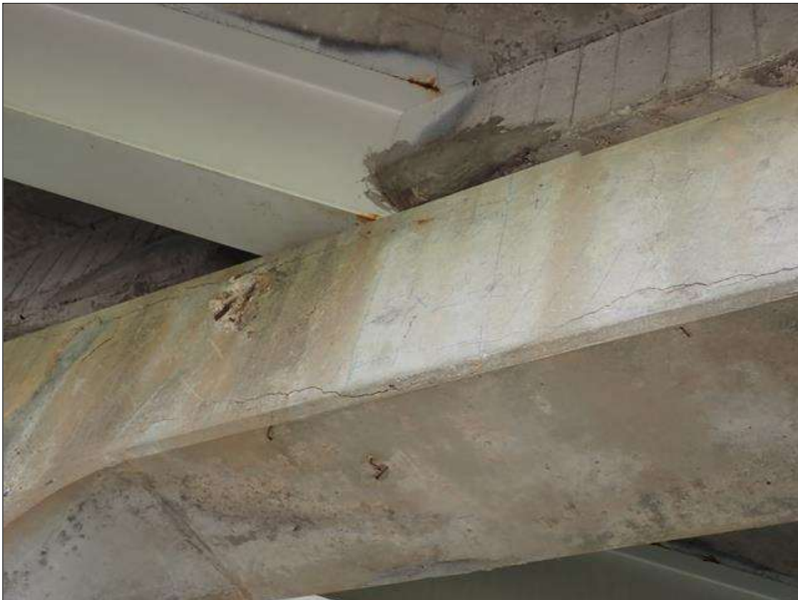
Bent 2 Cap 1: south and north faces of cap, multiple delaminations/spalls (up to 8 feet x 2 feet x 1.5 inch deep), some with exposed rusted rebar and associated cracks (up to 1/8 inch wide)
