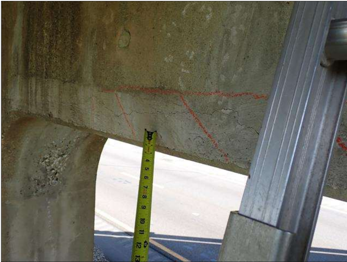
Bent 2 Cap 1: south and north faces of cap, multiple delaminations/spalls (up to 8 feet x 2 feet x 1.5 inch deep), some with exposed rusted rebar and associated cracks (up to 1/8 inch wide)
