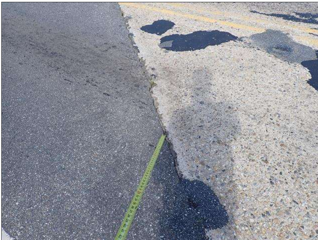
Span 1 Deck: along end bent 1, multiple edge spalls [up to 6 inches x 2 inches x 1 inch deep]
