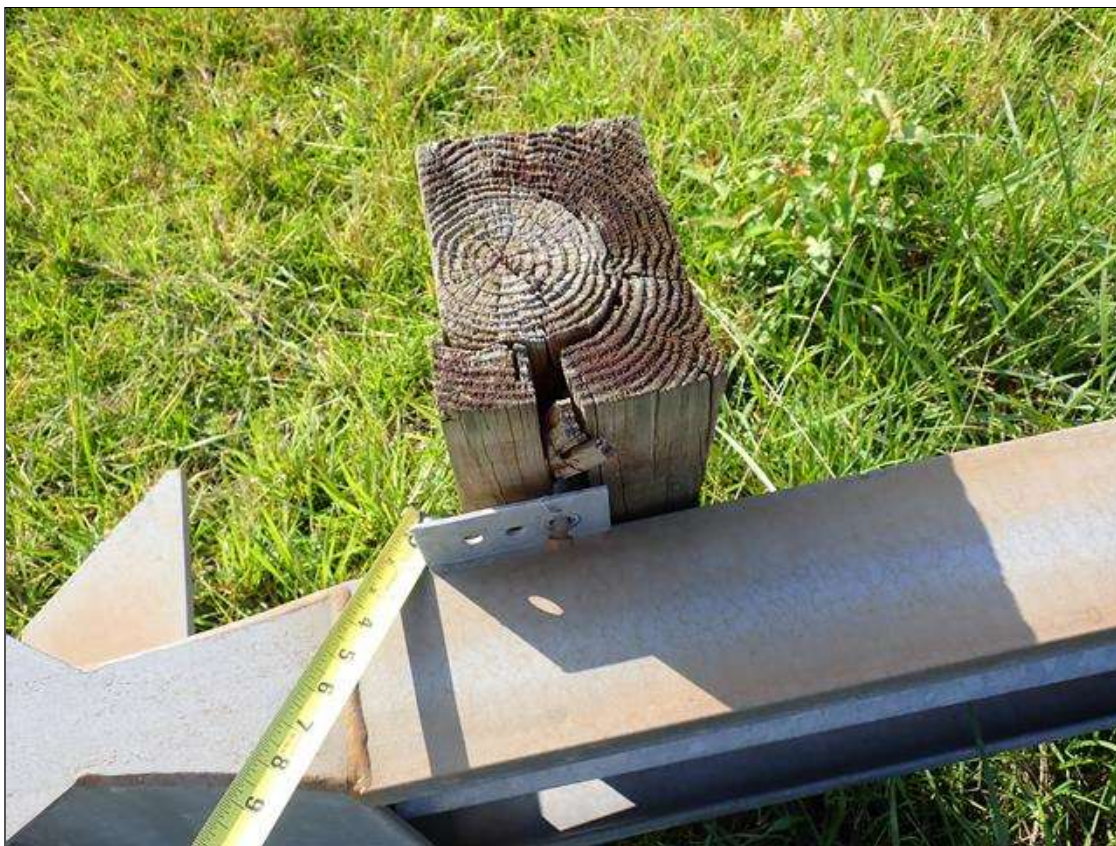
(PAR) northeast guardrail termination, end post split with disconnected termination block
