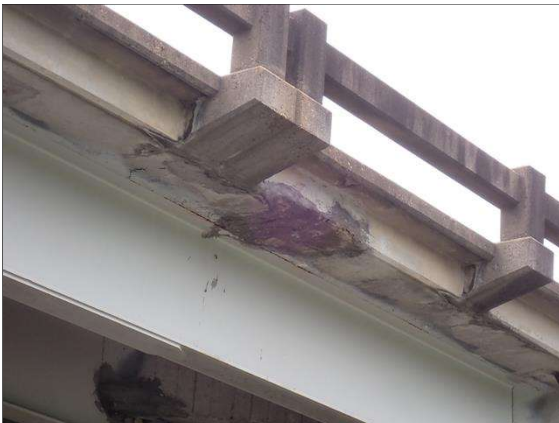
Span 3 Deck: [PAR] along left overhang, multiple failed patches with associated delaminations [up to 30 inch diameter] over traffic
