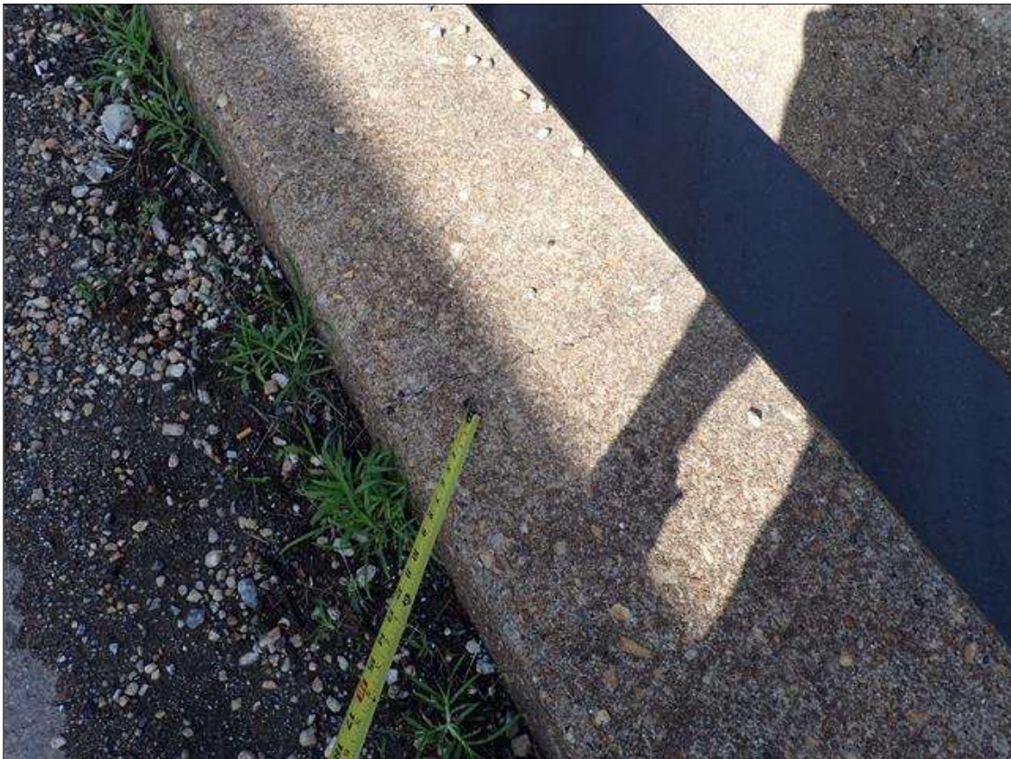
Span 3 Left Bridge Rail: along curb, wraparound vertical cracks [up to 1/32 inch]
