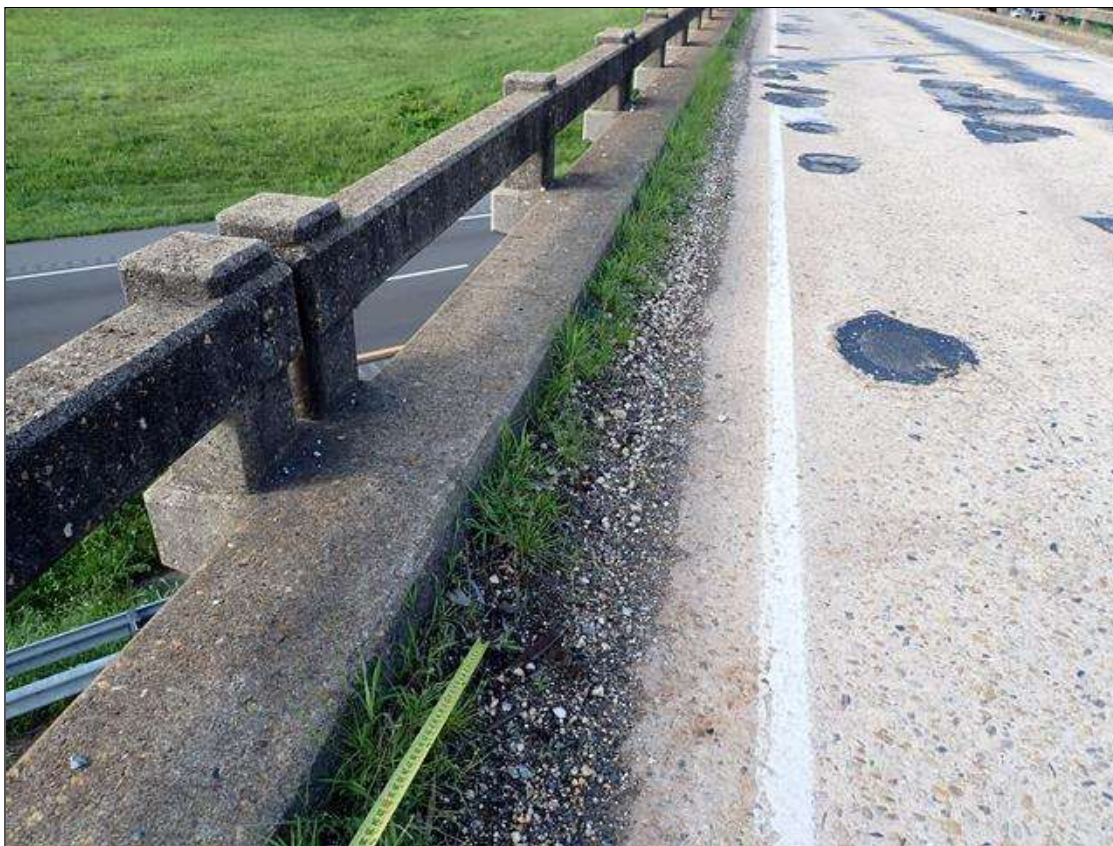
along the curblines, debris accumulation (up to 2 feet wide x 4 inches wide) with vegetation, with multiple clogged drains
