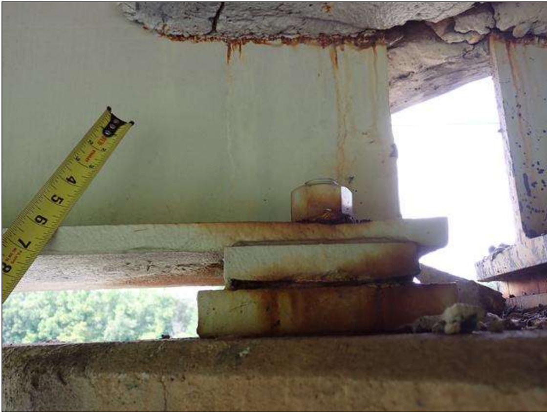
Span 2 Beam 1: (PAR) at bent 2, web adjacent to diaphragm, painted over section loss (3/8 inch average remaining x 6 inch x 1 inch); underside of bottom flange, painted over pitting (up to 1/8 inch deep x 6 inches) with corrosion reinitiated
