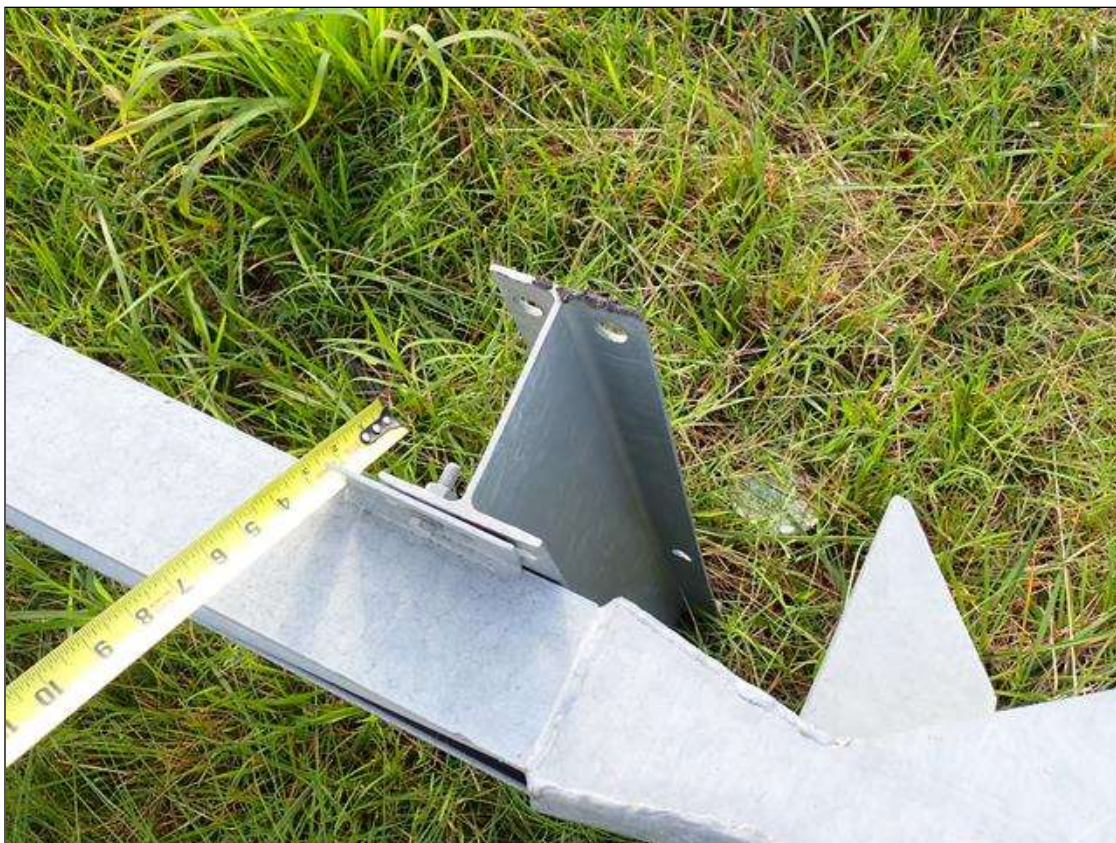
(PAR) southeast guardrail termination, impact damage with leaning end post
