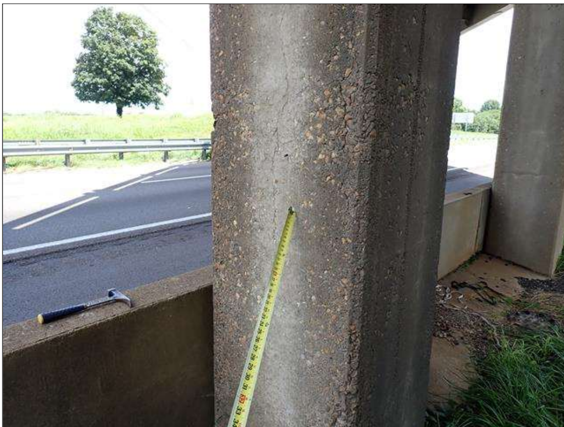
Bent 1 Pile 1: west face, near ground, poor consolidation (up to 5 feet x 1 foot x 1 inch deep) with associated vertical cracks (up to 1/8 inch wide x 3.5 feet)
