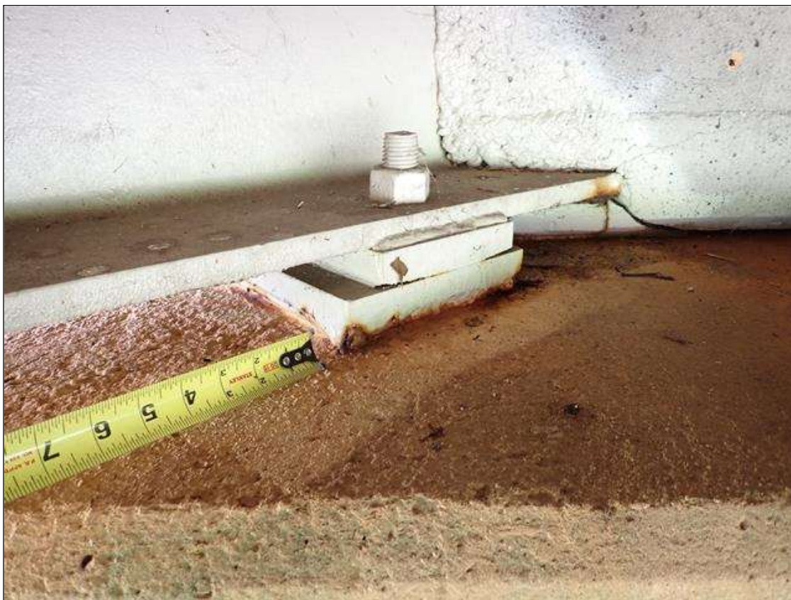
Span 1 Beam 4 - Near Bearing 4: painted over section loss (up to 1/8 inch deep) with corrosion reinitiated
