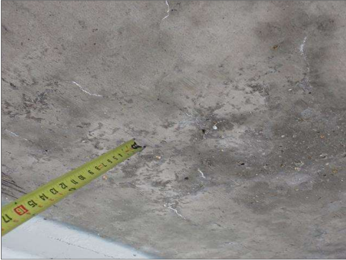
Span 1 Deck: throughout underside of deck, areas of map cracks (hairline), some with efflorescence at random
