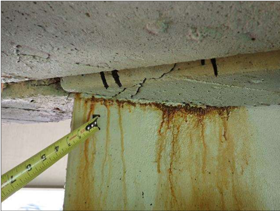
Span 3 Beam 3: (PAR) at bent 3, web adjacent to diaphragm, corrosion with section loss (3/8 inch average remaining x 13 inch x 1.5 inch)
