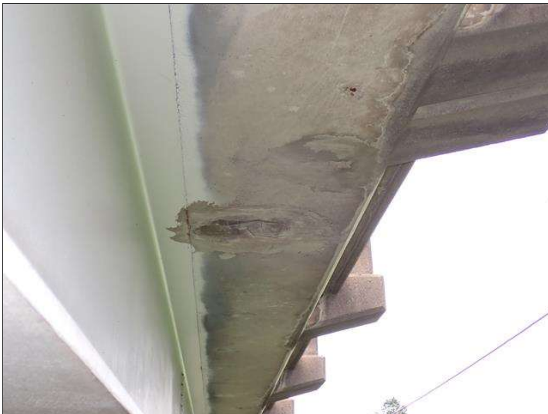
Span 4 Deck: SPAN 4 BOTTOM OF LEFT OVERHANG HAS multiple failed PATCH AREAS/DELAMINATIONS (up to 2 feet x 15 inch) THROUGH OUT THE SPAN
