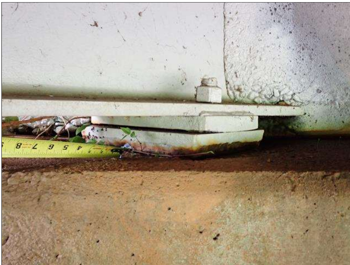
Span 4 Beam 1 - Far Bearing 1: painted over section loss (up to 3/16 inch deep) with corrosion reinitiated
