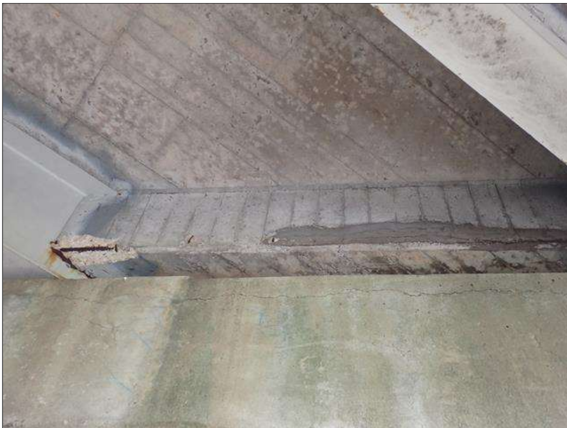
Span 3 Deck: at bents 2 and 3, end diaphragm, in all bays, spalls/delaminations/unsound patches (up to 5 feet x 6 inch x 2 inches deep) with exposed rusted rebar
