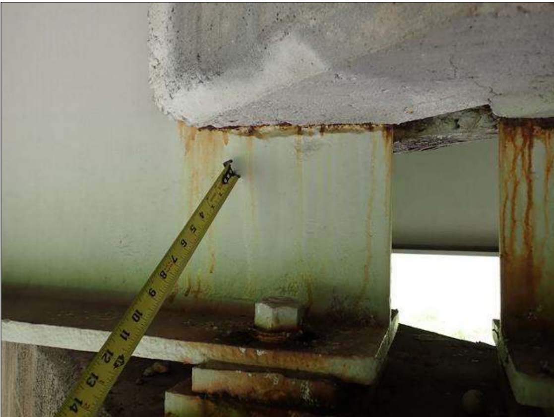
Span 2 Beam 3: (PAR) at bent 2, web adjacent to diaphragm, painted over section loss (5/16 inch average remaining x 9 inch x 1 inch); lower web, painted over pitting (up to 1/8 inch deep x 3 inch x 3 inch) with corrosion reinitiated
